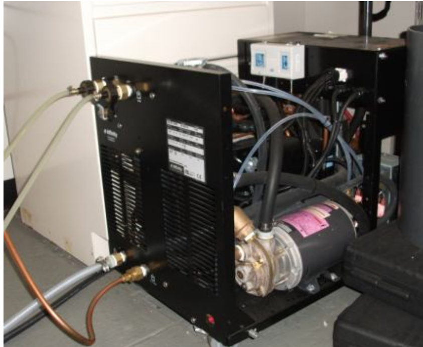
Fig. 2.8 Cooling system for our sputtering system.
