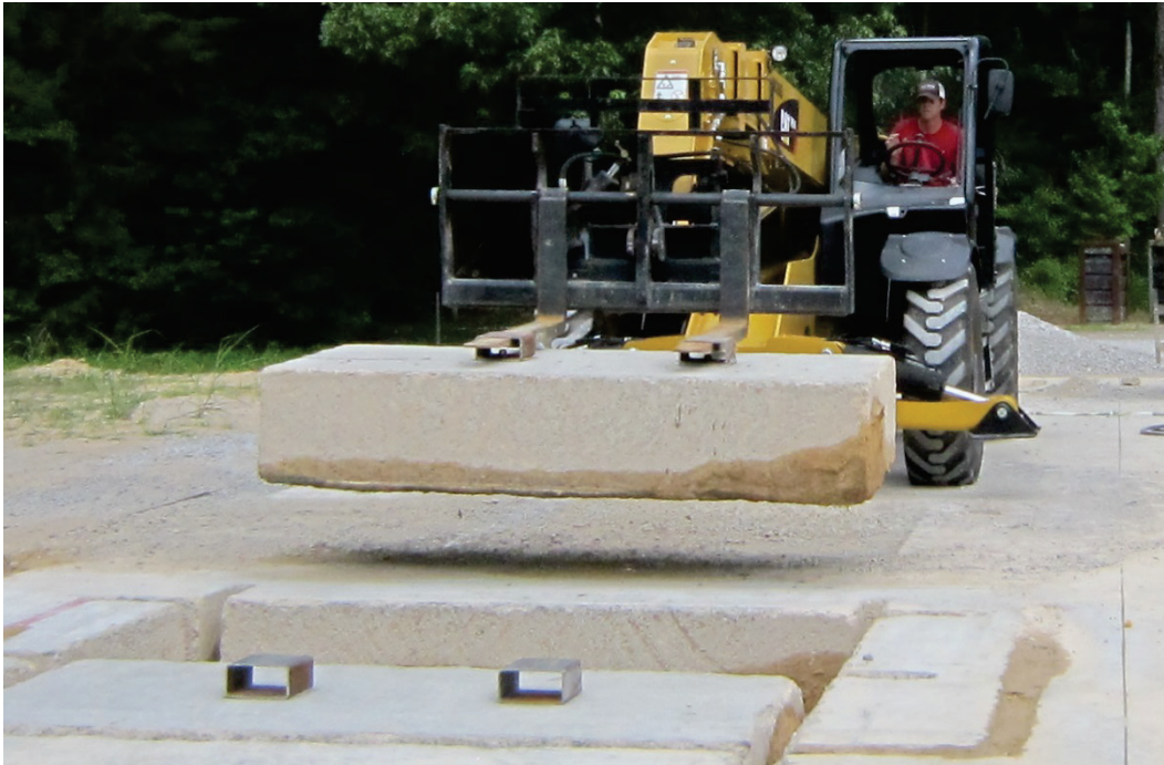
Figure 55. Successful removal of PCC using the box beam with all thread rod.
