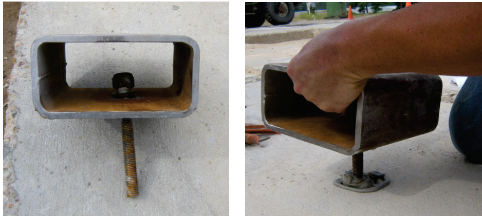
Figure 53. All thread rod with nut, inserted through opening on the bottom of the box beam and placed into drilled hole in PCC.
