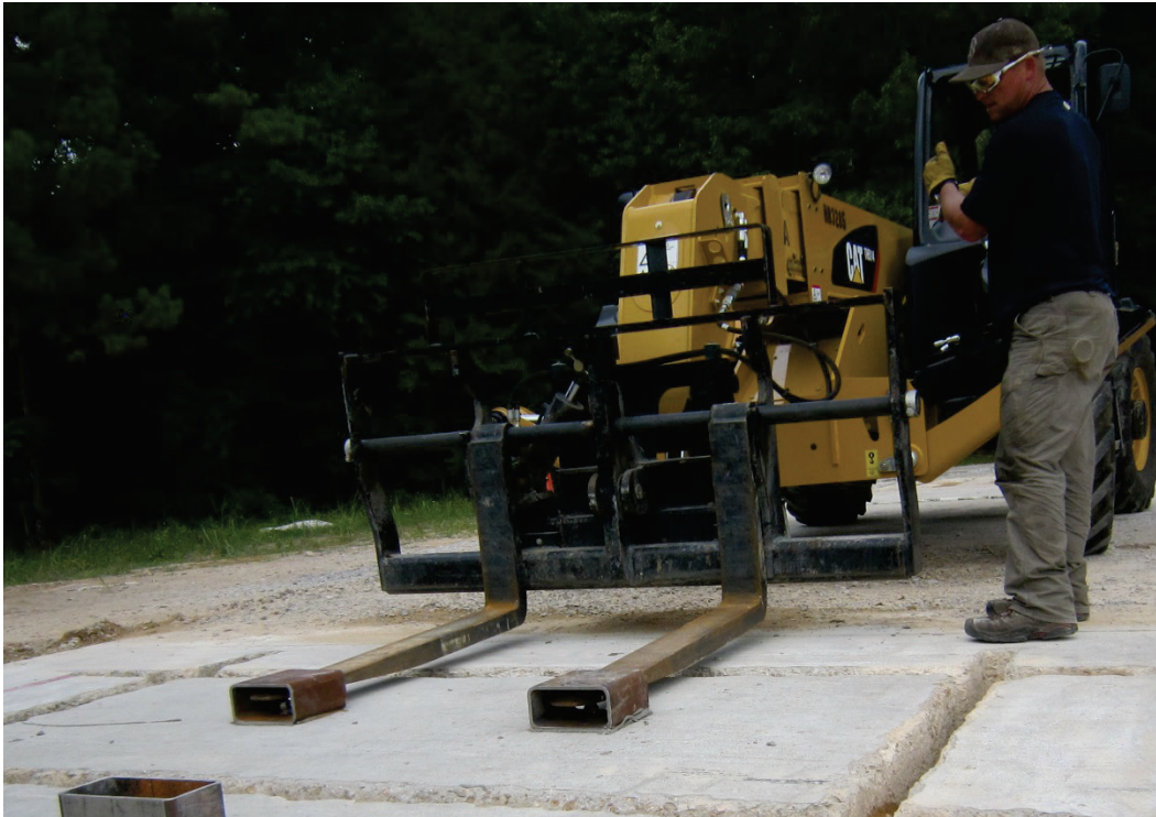
Figure 54. Placing the telehandler forks into the box beams attached with all thread rods with bolts and nuts.
