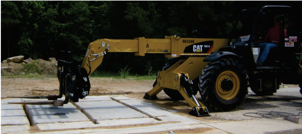
Figure 51. Epoxy on pavement failed to hold.
