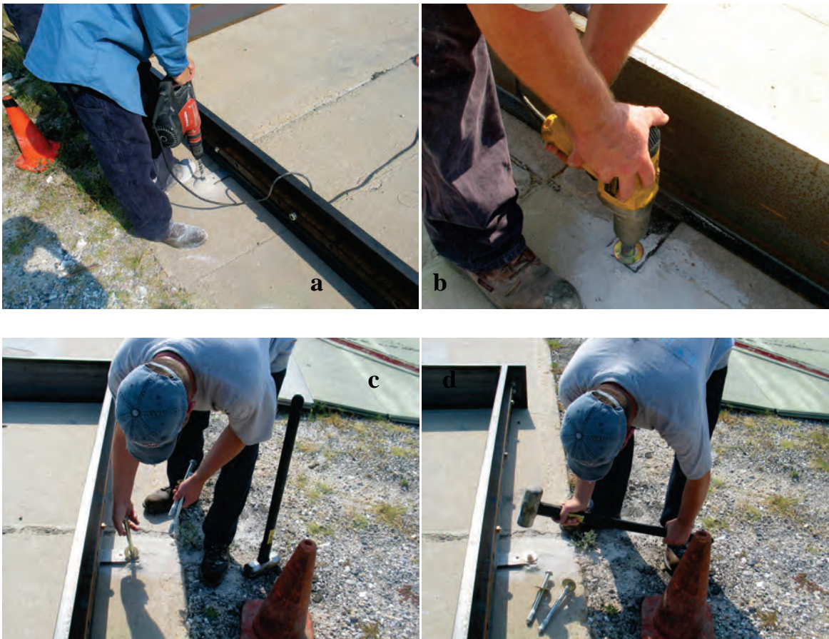
Figure B.6. Securing formwork to solid surface: (a) drilling anchor hole, (b-d) installing and activating the anchor.
