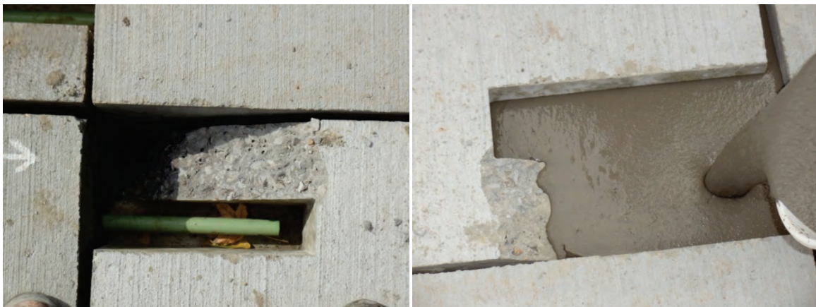
Figure D.4. Damaged and repaired dowel bar receptacle on panel 4.
