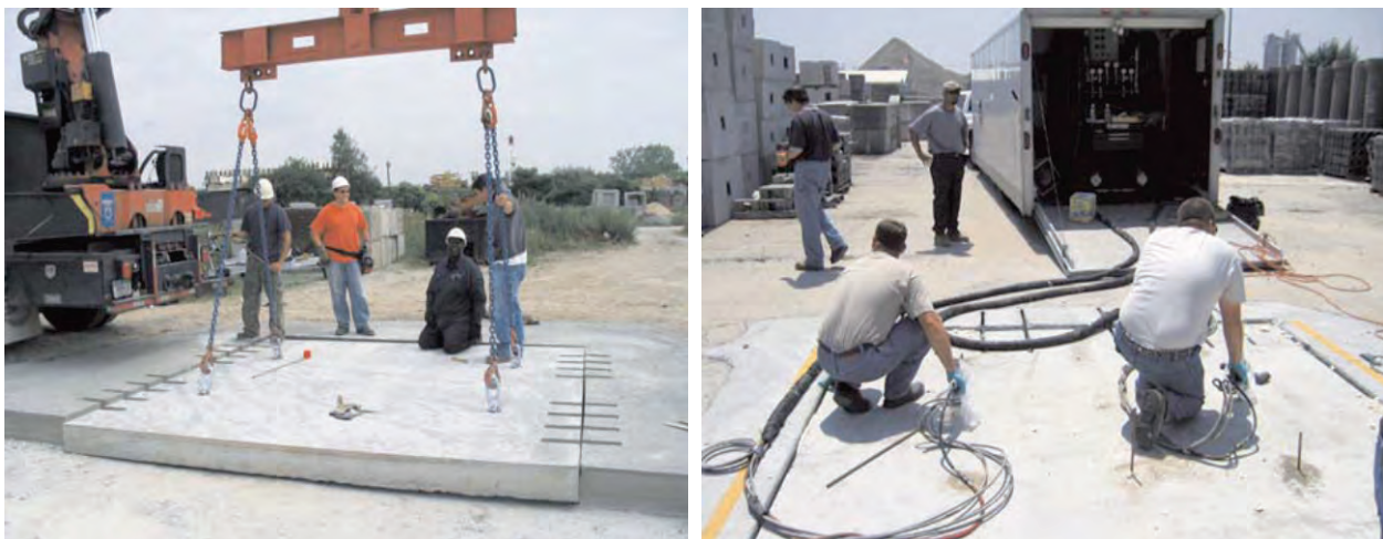
Figure A.9. (Left) installing Roman Road slab; (right) injecting polyurethane foam (Roman Stone Construction 2012).
