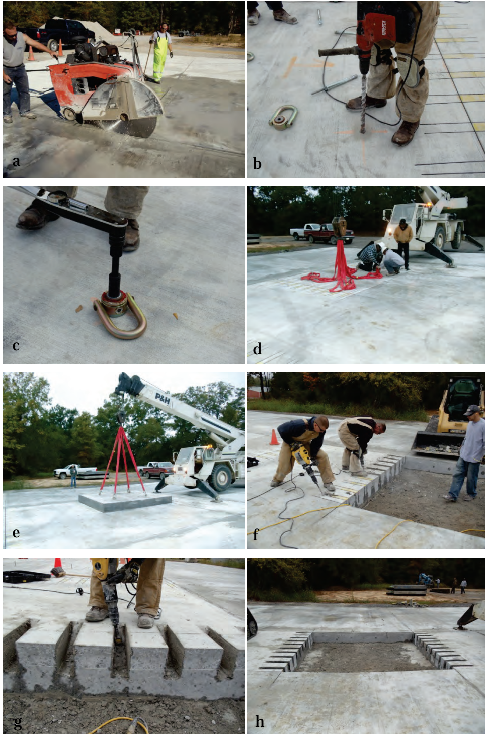
Figure C.4. Preparation and removal of parent PCC: (a) saw cutting dowel receptacles and repair area, (b) drilling to install concrete lifting anchors, (c) installing lifting eyes, (d) connecting lifting eyes to crane rigging, (e) lifting “damaged” pavement, (f) preparing dowel receptacles using jackhammers, (g) close-up of dowel receptacles, and (h) prepared repair area.
