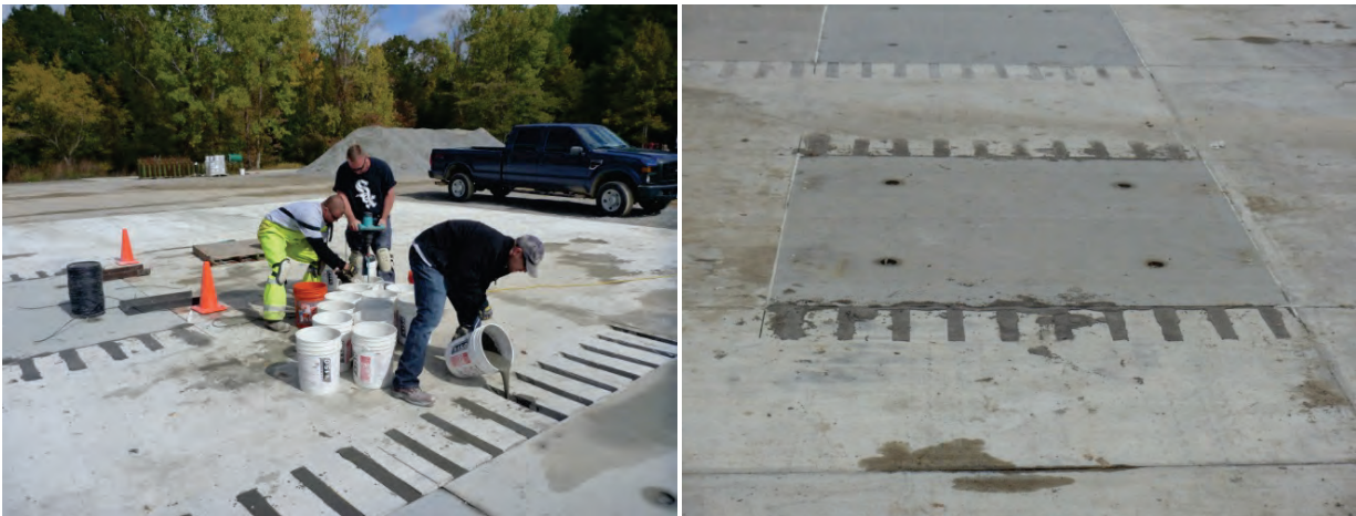
Figure C.8. Left: placement of rapid-setting grout in dowel receptacles, and right: grouted and sealed panel.
