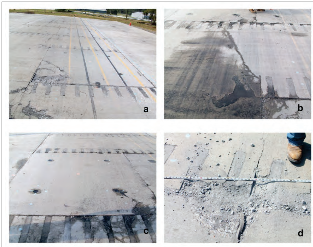
Figure 3.5. Repair failure details: (a) Repair 1, Panel 1: high-severity corner break/spall and shattered parent slab; (b) Repair 2: diagonal cracking in parent slab between Repairs 1 and 2 and cracking and spalling of Panel 2 due to the parent slab deterioration; (c) close-up of the cracking and deterioration in the parent slab and dowel slots and corner of Panel 2; (d) Repair 3, Panels 6 and 7: high-severity spalling in corner of Panels 6, 7, and the parent slabs south of the repair.
