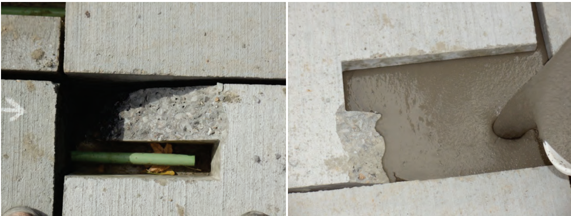
Figure C.11. Left: broken corner of a panel, and right: repair of broken corner.
