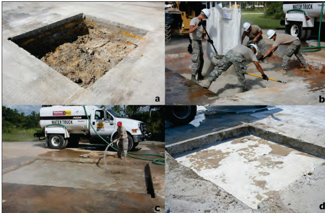
Figure 6.5. (a) Prepared repair, (b) backfilling with flowable fill, (c) adding water, (d) cured backfill surface after 15 min.
