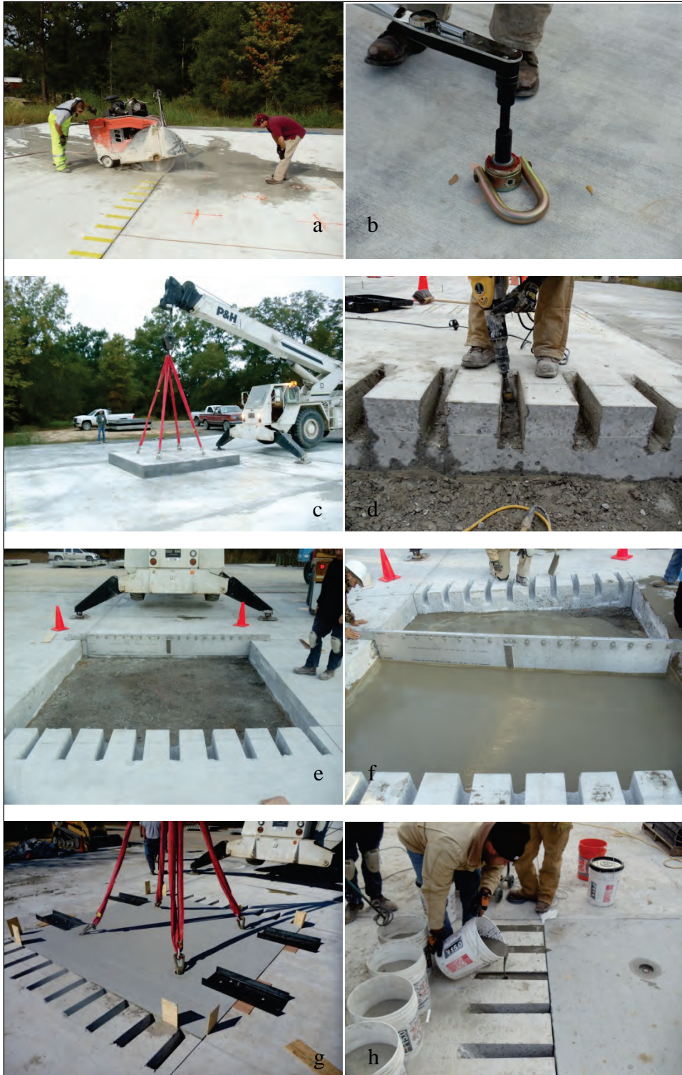
Figure 4.2. Repair procedure: (a) saw cutting the repair area and dowel slots, (b) installing lifting eyes to concrete expansion anchors, (c) removing parent PCC, (d) preparing dowel slots, (e) prepared repair area, (f) screeding flowable fill bedding material, (g) lowering panel into repair area, and (h) sealing dowel slots with rapid-setting grout.
