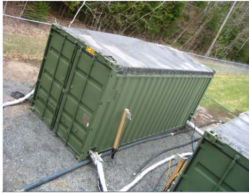
Figure 76: GE deployable MBR/RO wastewater treatment system.
