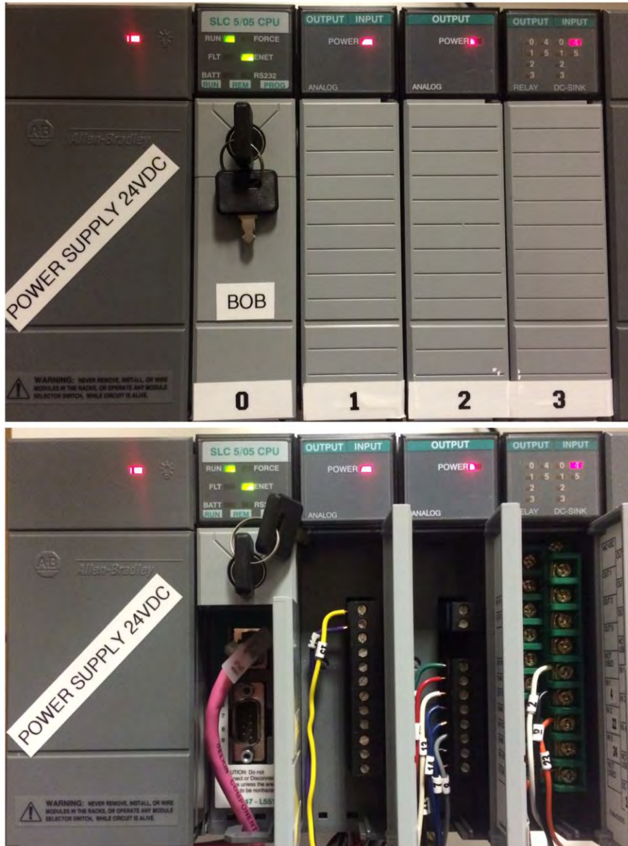
Figure 10. PLC I/O modules their slot locations 0–3 (left to right)
