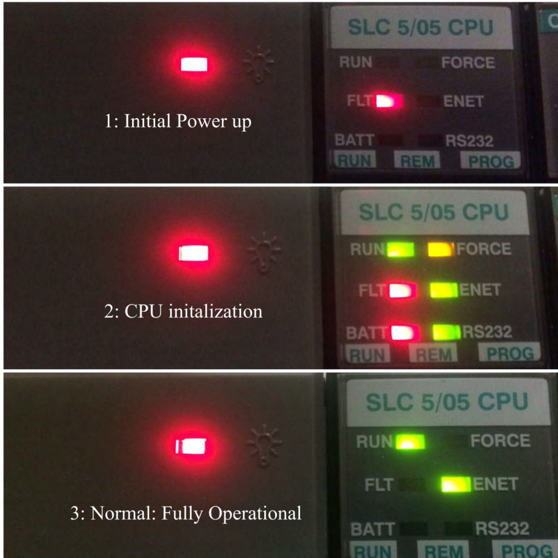
Figure F16. Sequence of indications on the PLC as it powers up
