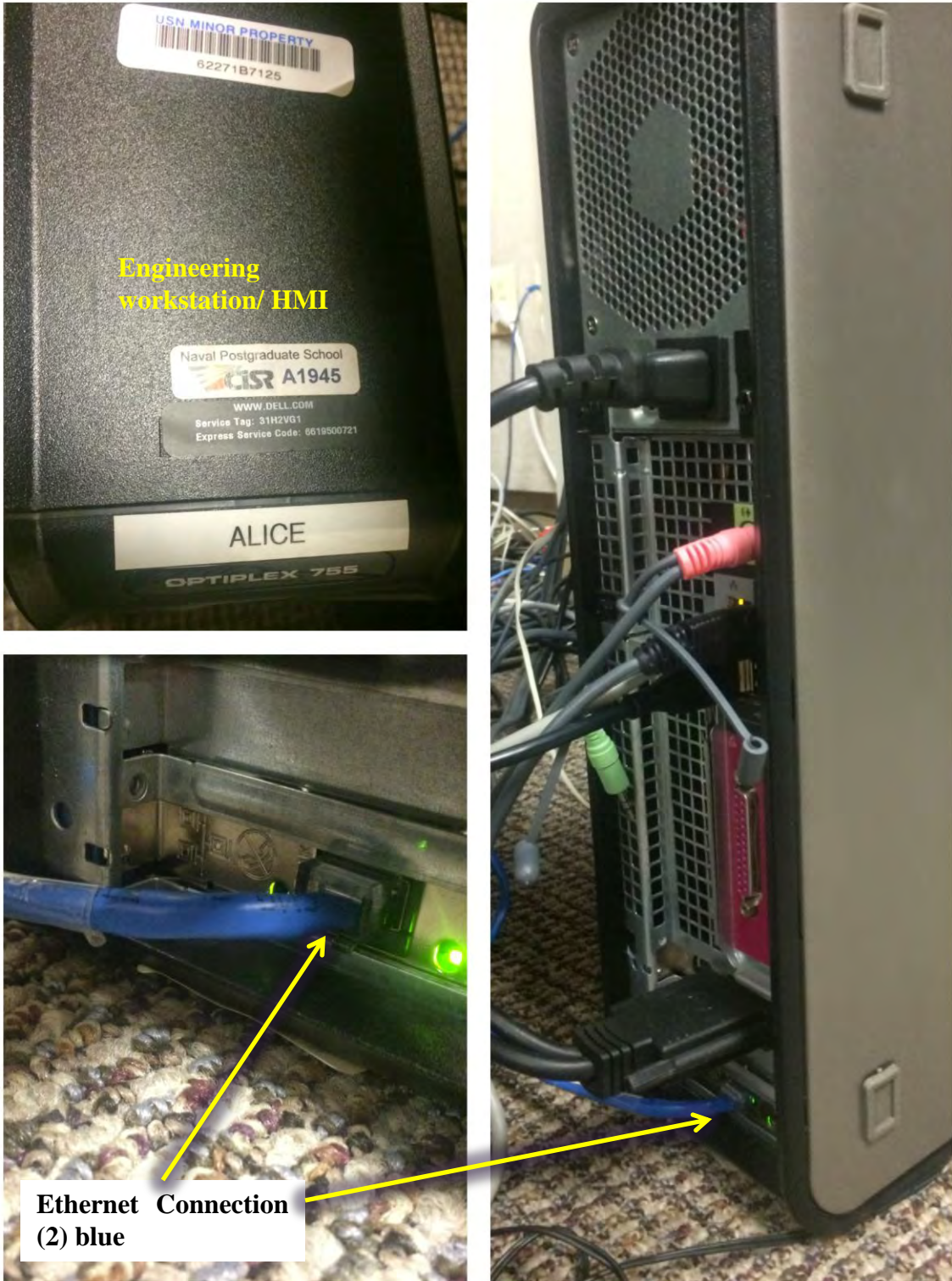
Figure F3. Engineering workstation and HMI
