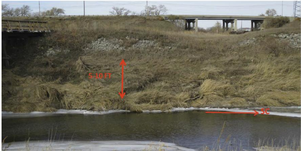
Area 15, Station 211+00. This area is located approximately 3,000 feet north of “O” street between two railroad bridges and the photo shows channel bank erosion along approximately 100 feet of the left descending bank. The proposed repair would consist of reshaping the levee and replacing lost bank material with compacted, non-dispersive clay and riprap or building a landside piggy back levee if space is available.
