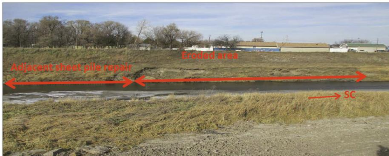
Area 16, Station 280+00. This area is located directly west of the Antelope Valley Parkway Bridge and the photo shows channel bank erosion along approximately 200 feet of the left descending bank. The proposed repair would consist of reshaping the levee and replacing lost bank material with compacted, non-dispersive clay and riprap and stabilizing an area with sheet pile to match the adjacent flood repair.
