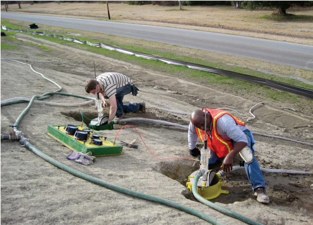
Figure 16. The ERDC team performing a field JET test on the lime-treated segment of the levee.
