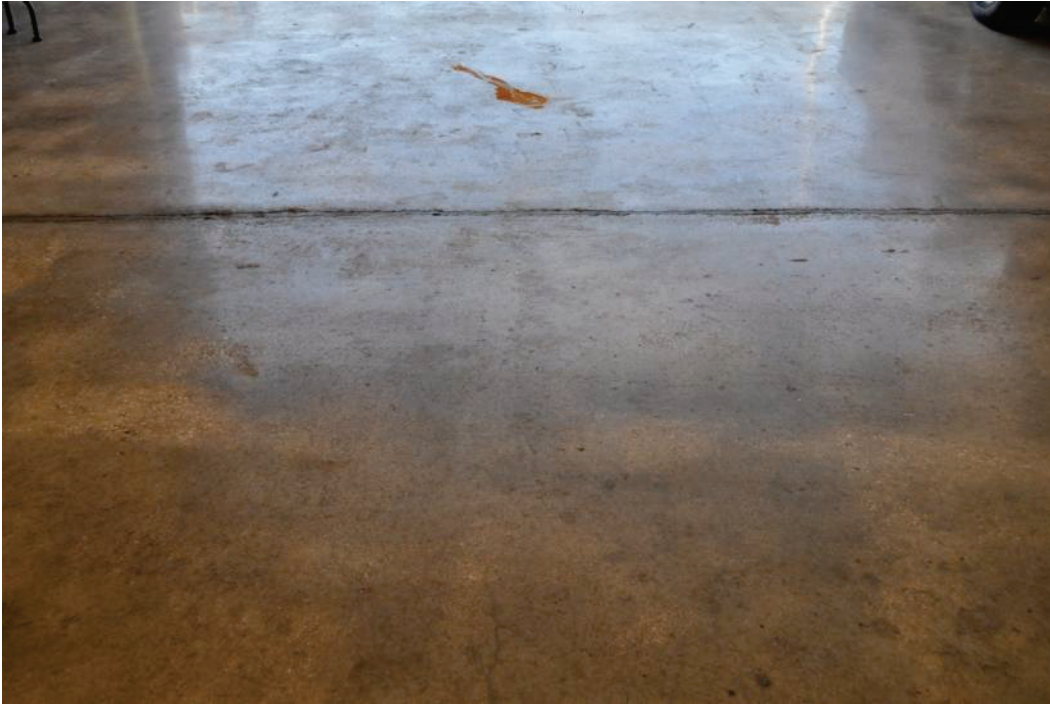
Figure 23. General floor condition at 9 months.
