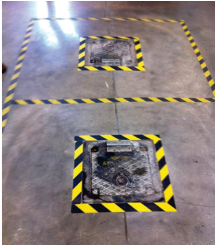
Figure 22. Safety striping tape marking junction boxes on floor.
