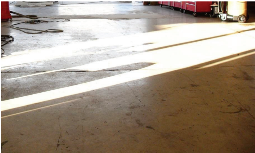
Figure 2. Condition of epoxy-coated maintenance bay floors before project.
