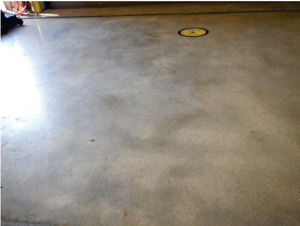
Figure 25. Bay 4 floor surface area after 1 year of service.
