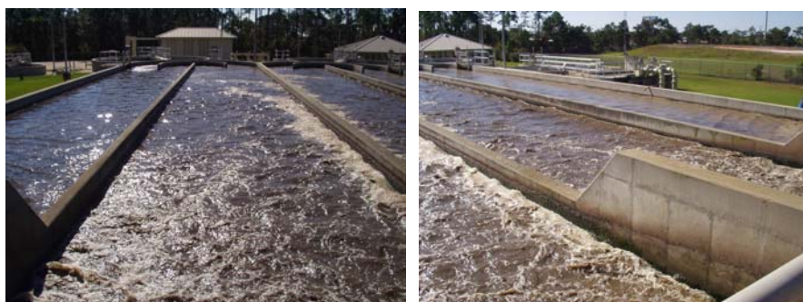
WWTP Aeration Basins
