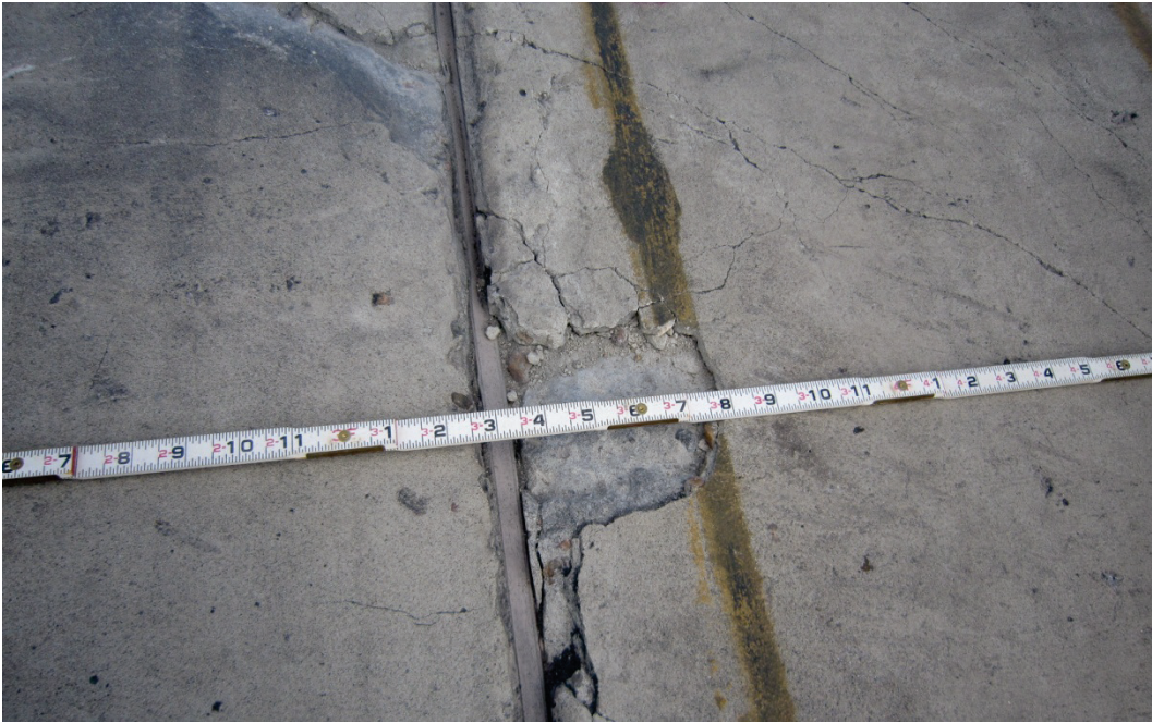
Figure 65. Crater 2, 900 passes, high-severity joint spall.
