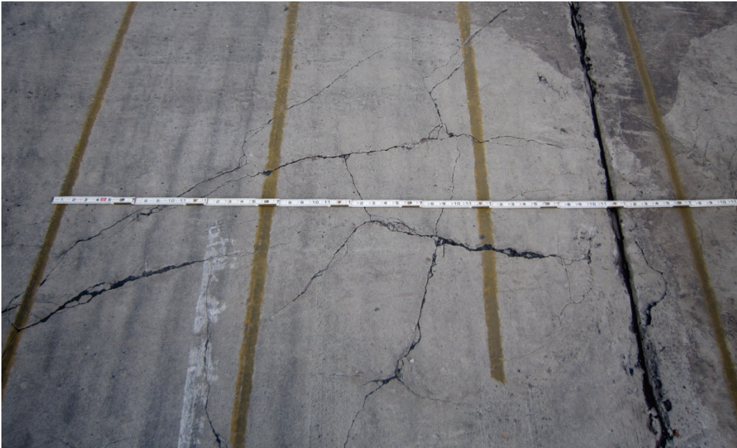
Figure 64. Crater 2, 900 passes, medium-severity cracking.
