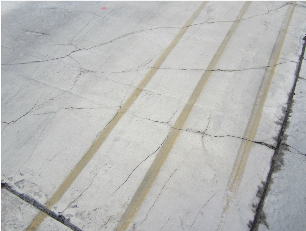
Figure 66. Crater 2, 1,500 passes, medium-severity longitudinal cracking.
