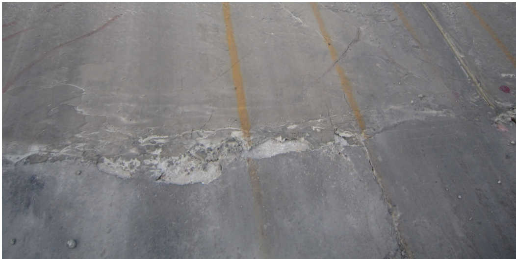
Figure 68. Crater 3, 100 passes, medium-severity joint spall.
