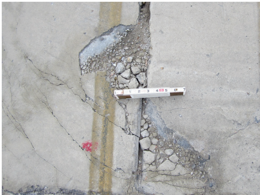
Figure 67. Crater 2, 1,500 passes, high-severity joint spall.
