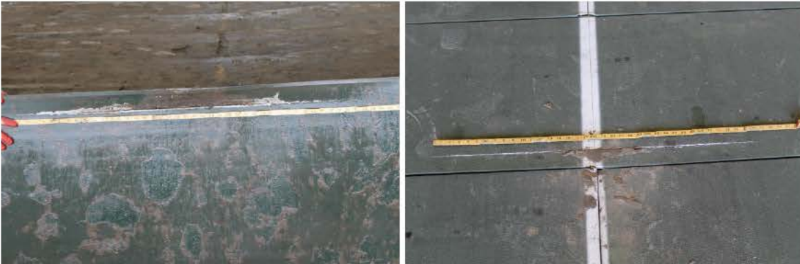
Figure 31. Crack on bottom (left) and top (right) surface of I-11.
