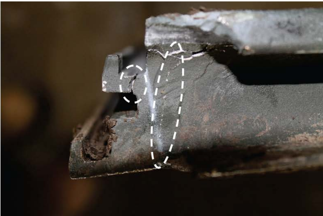
Figure 37. Cracked upper underlap rail and hairline crack at weld of I-54.
