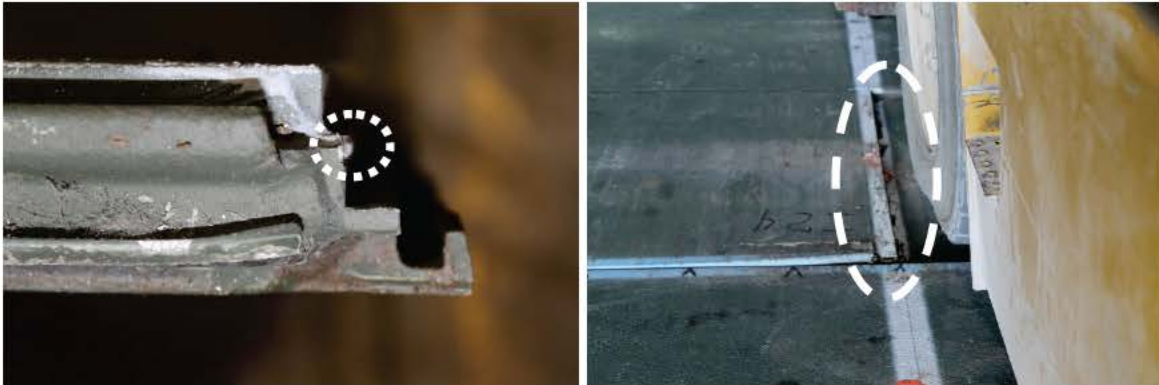
Figure 27. Broken upper underlap rail I-79 (left) and I-25 (right).
