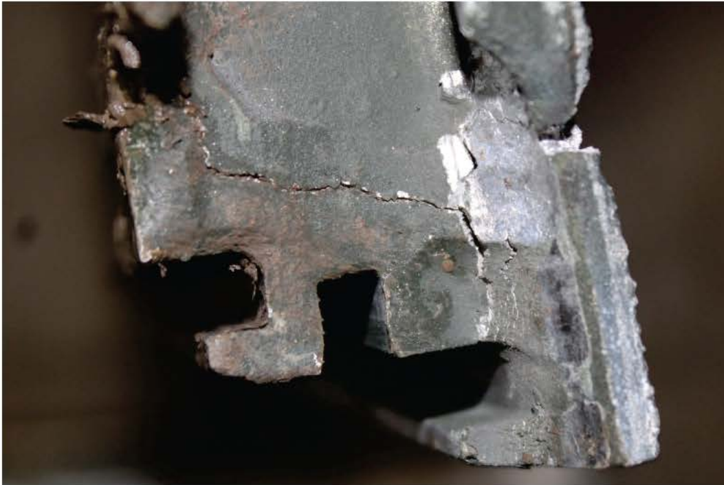
Figure 36. Crack at weld of I-62.
