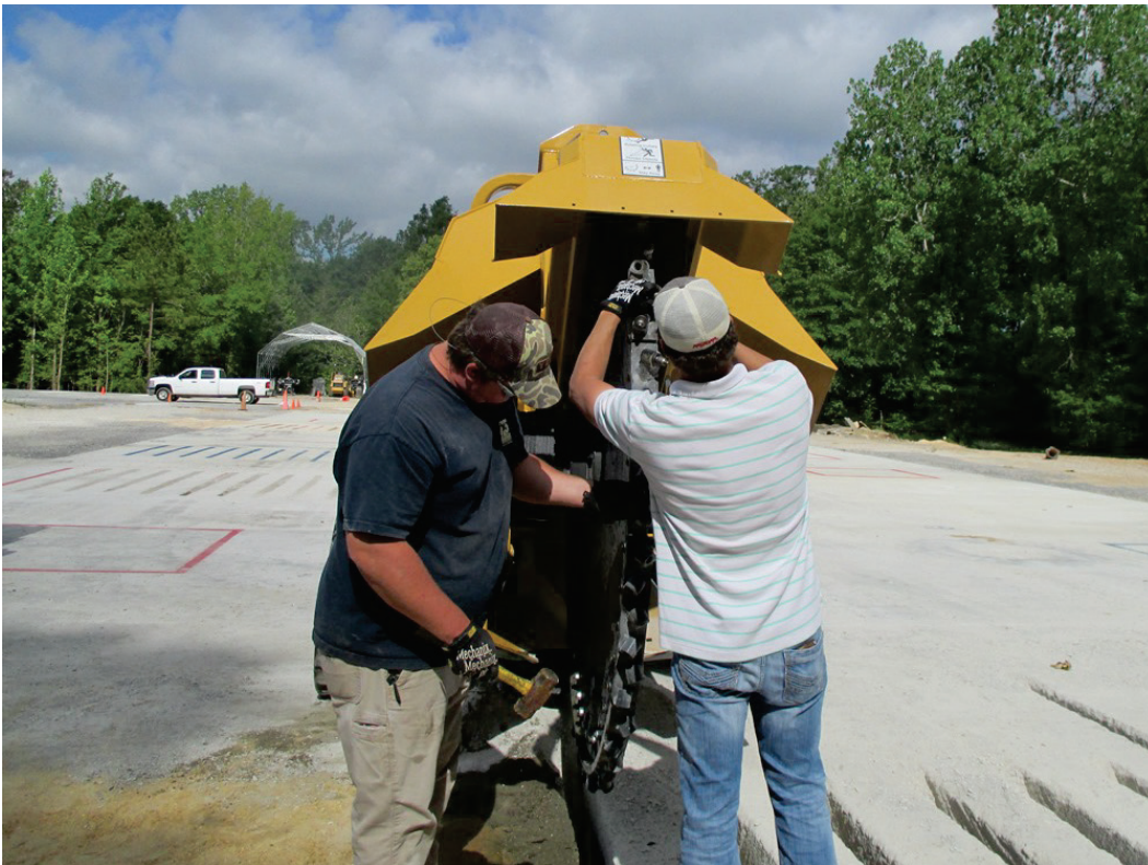
Figure 21. Replacing teeth on a Vermeer RW1236W saw.
