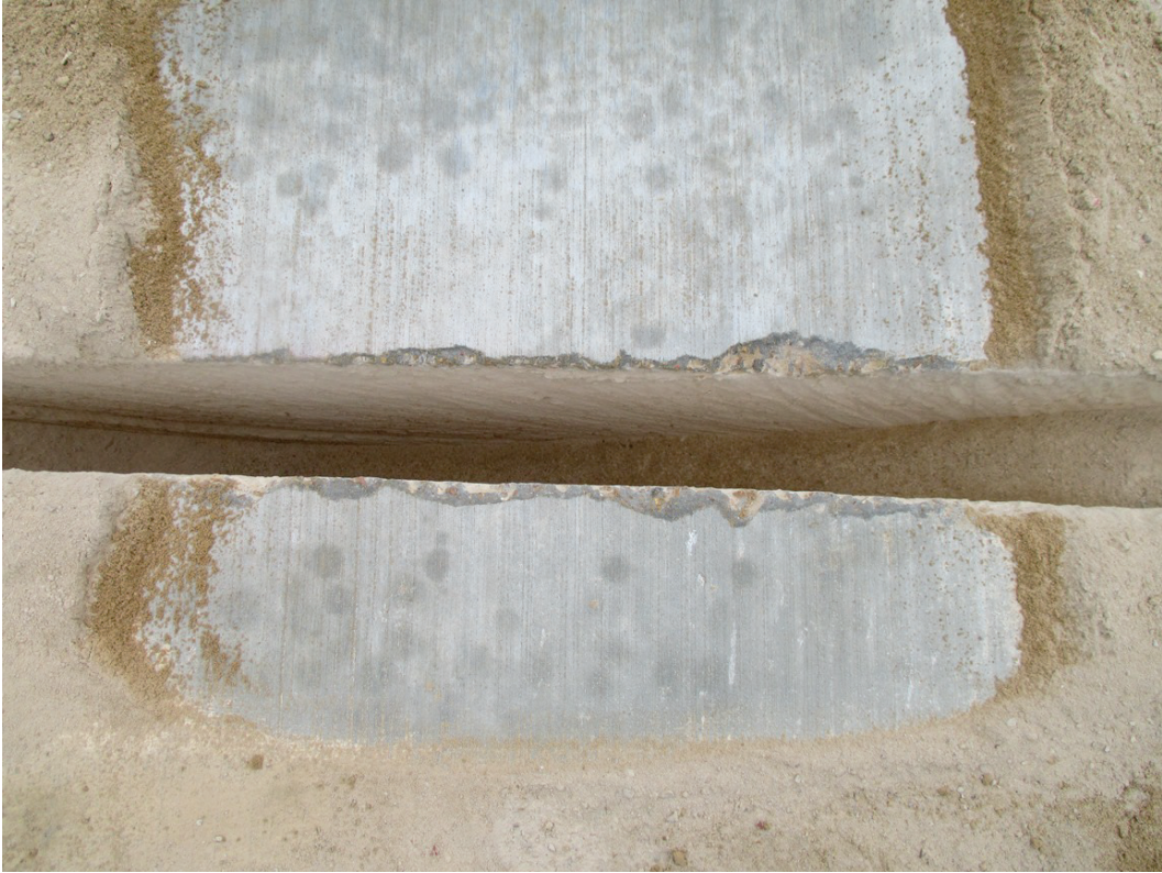
Figure 49. Spalling of chert PCC from Kennametal RP15 teeth on CAT SW60.
