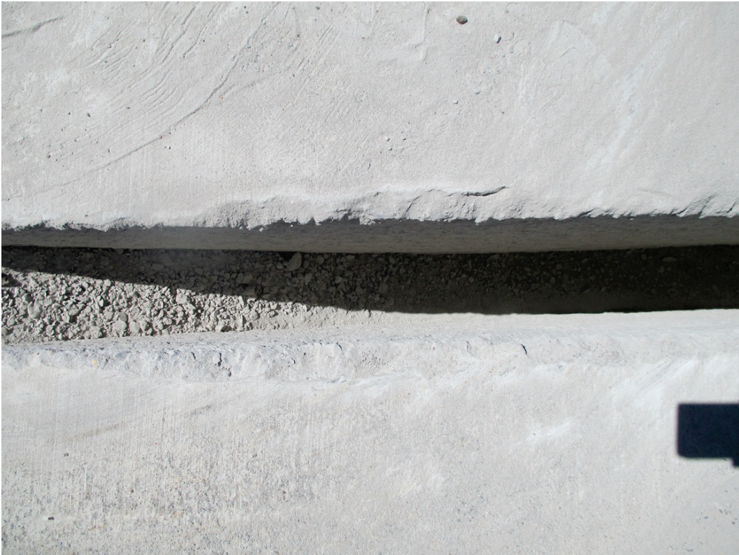
Figure 51. Spalling of limestone PCC with Kenn SM04 teeth on Vermeer RTX1250.
