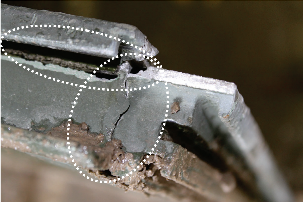
Figure 66. Damage noted in Panel 101 after removing from test section.
