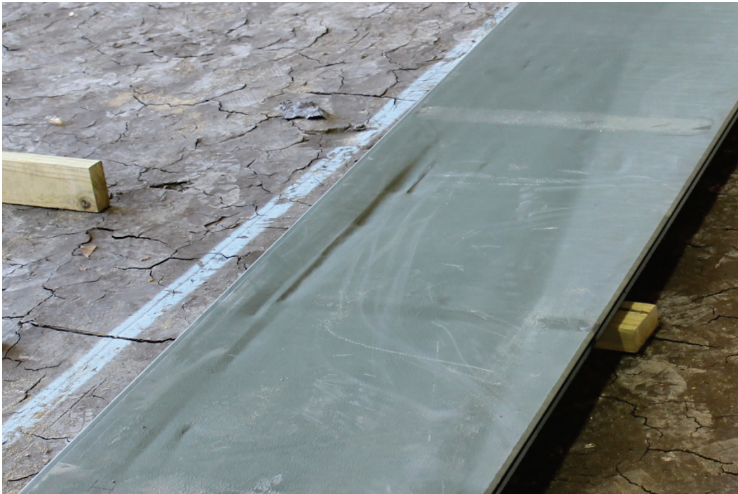
Figure 2. Damage noted on refurbished AM2 panel before applying traffic.
