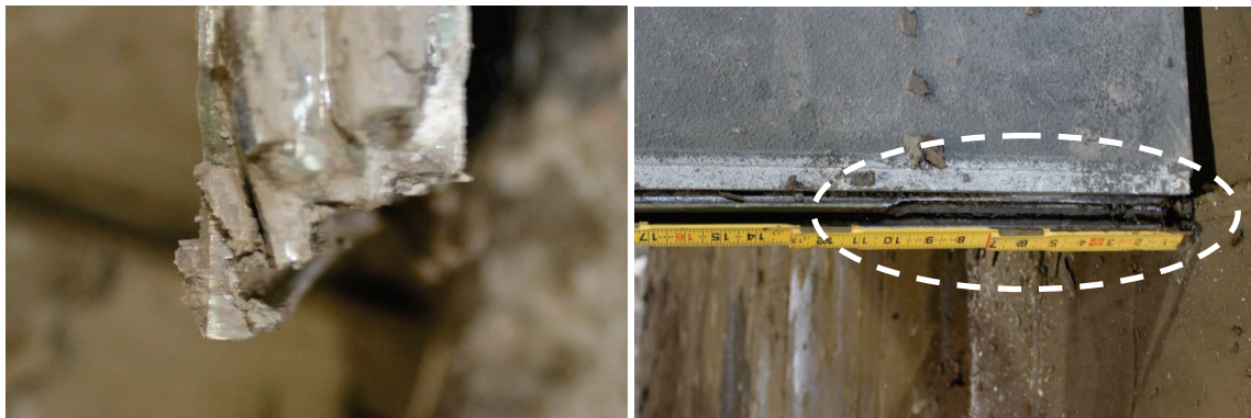
Figure 27. Upper underlap rail breakage at J46 (left) and J70 (right).
