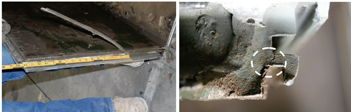
Figure 28. Lower overlap rail breakage at J69 (left) and J9 (right).
