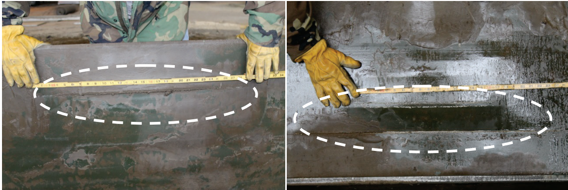
Figure 31. Cracks on bottom skin of J65 (left) and J62 (right).
