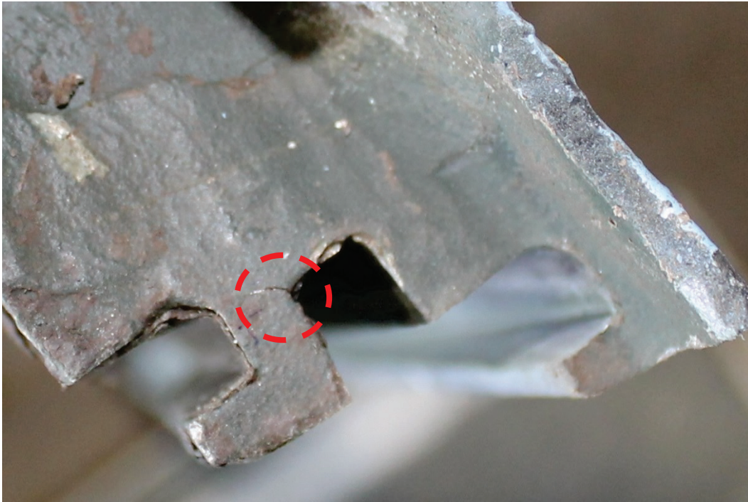
Figure 3. Crack initiation at lower overlap rail.
