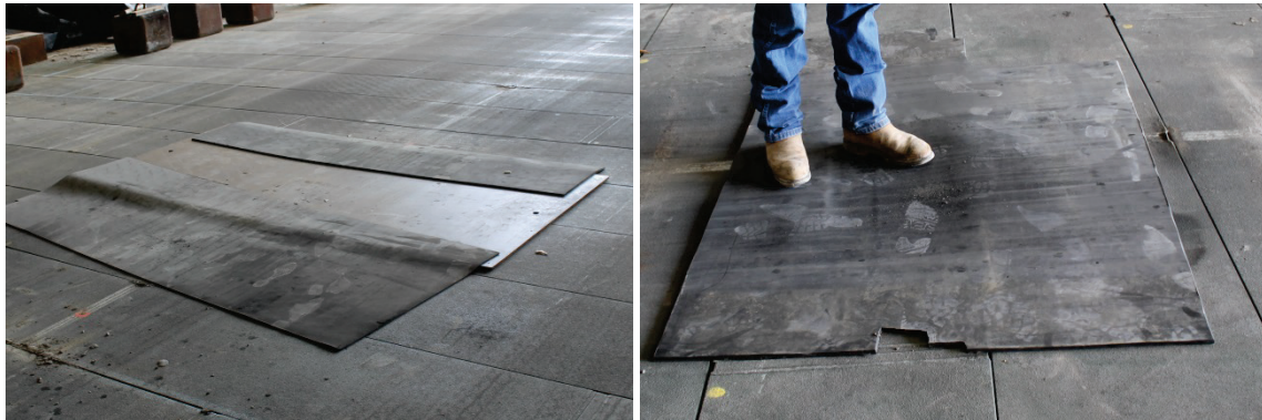
Figure 29. Metal plate placed on J46/J45 (left) and rubber mat placed on J74 (right).
