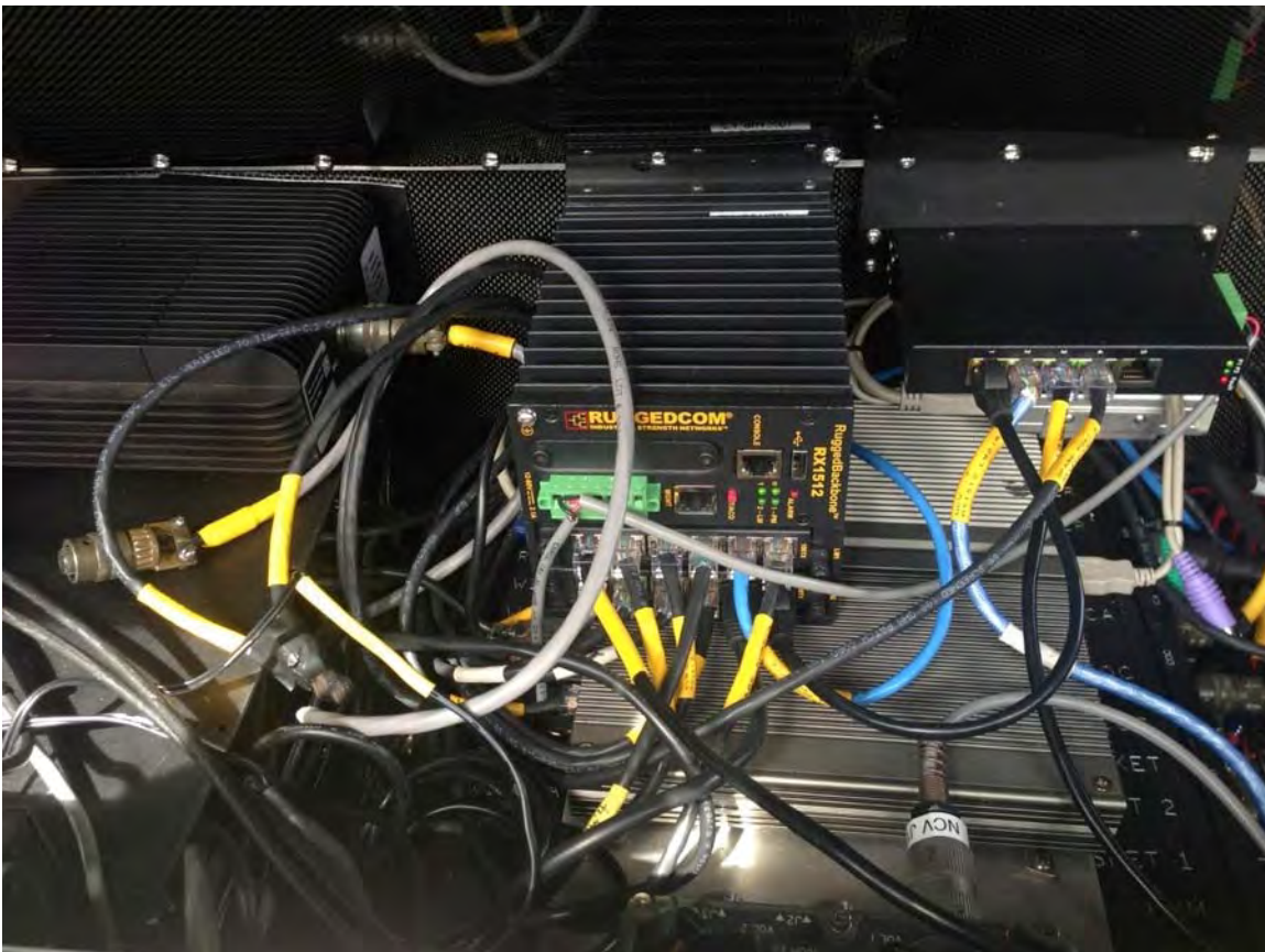
Figure 17. ME-L Internal Servers and Network Management
