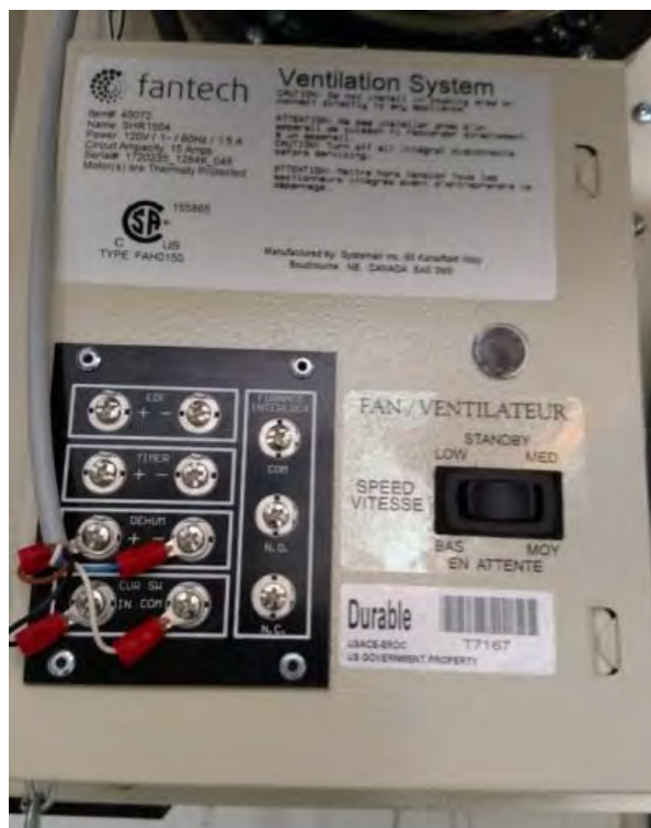
Figure 5-6. Fantech SHR 1504 HRV electrical panel.
