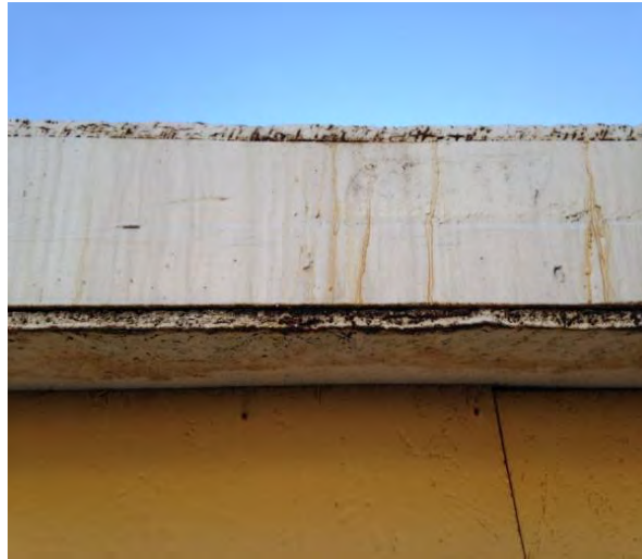
Figure 6-7. Deterioration of the edges of the SIP OSB panels on roof eave fascia.
