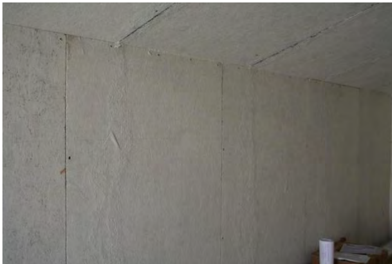
Figure 6-2. Water soaked into OSB panels from leakage (14 March 2014).
