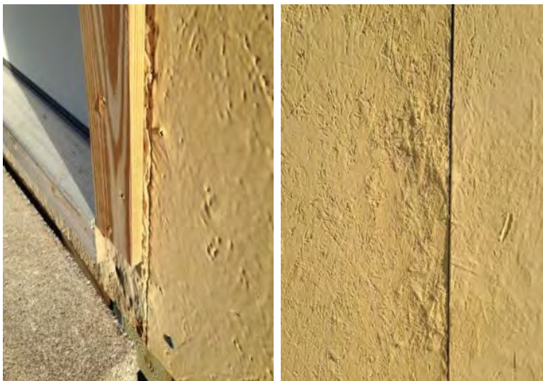
Figure 6-6. Separation of OSB strands in SIP hut panels.
