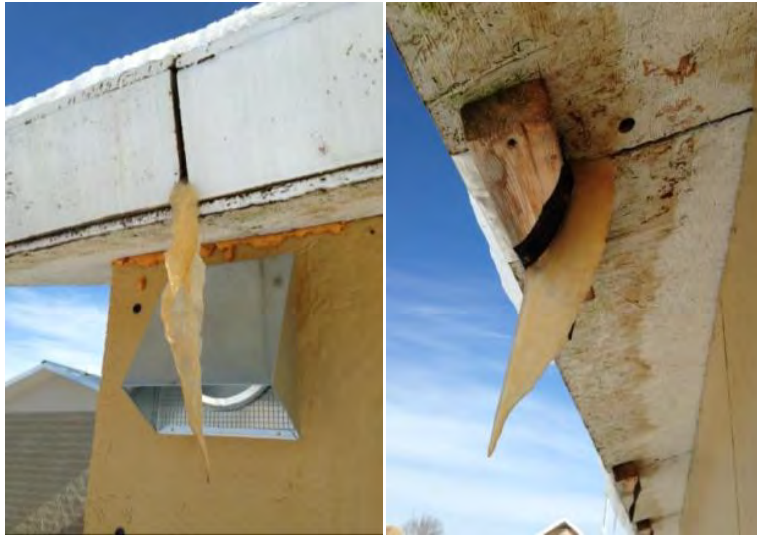
Figure 6-4. Icicles on seams with sealant (left) and tape (right).
