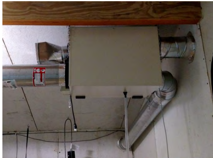
Figure 5-5. Fantech SHR 1504 heat recover ventilator installed in ERDC-CERL SIP hut.
