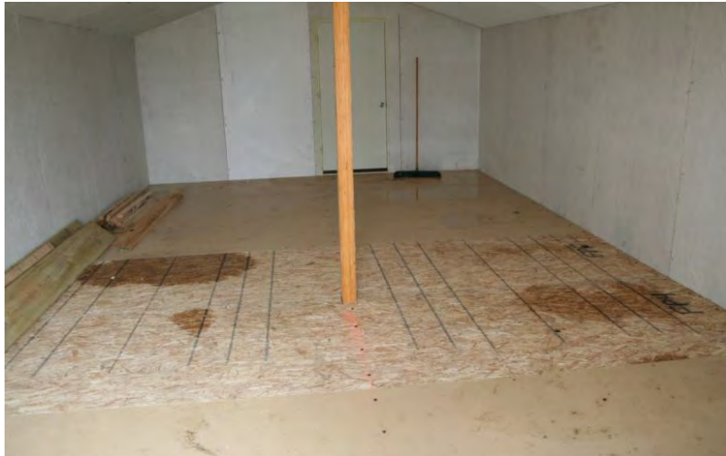
Figure 6-1. Standing water in SIP hut (14 March 2014).
