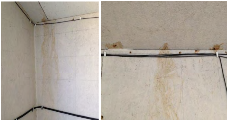
Figure 6-5. Staining on walls from water infiltration.
