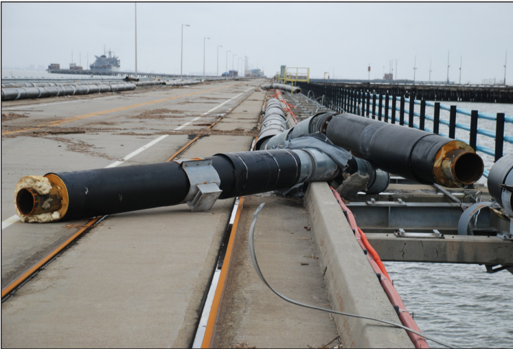
Destroyed by Hurricane Sandy
