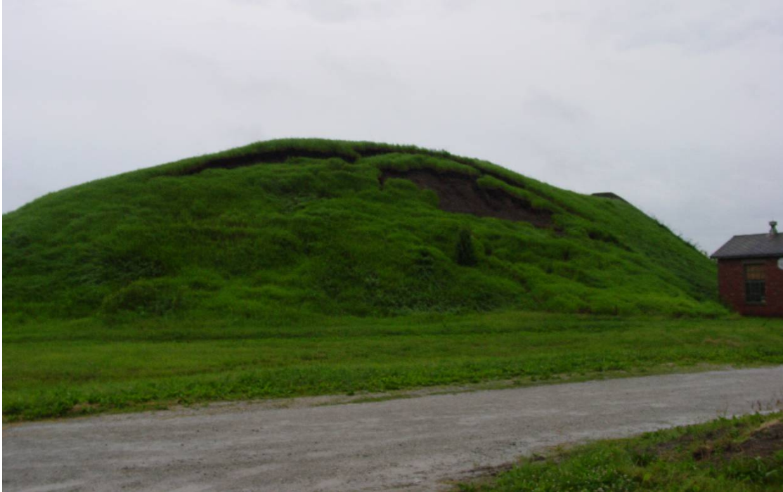
Figure 2. West face of Berm 3A-5-01 at Iowa Army Ammunition Plant showing evidence of erosion, vegetation loss, soil slope degradation and loss of protective height
