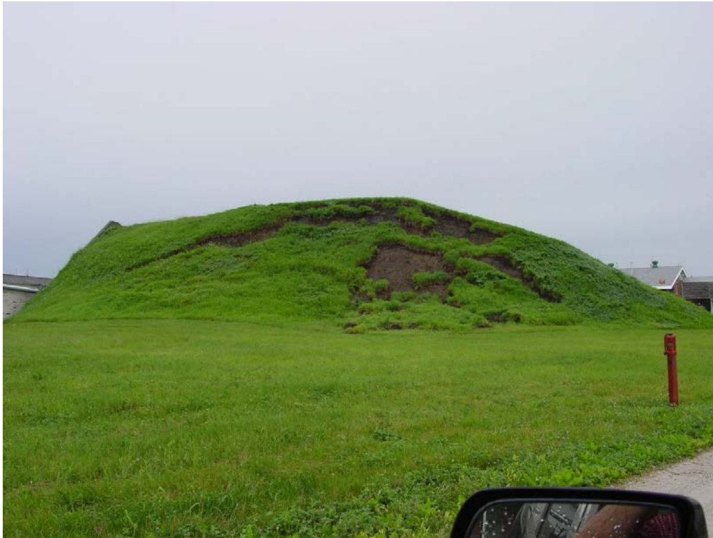
Figure 1. East face of Berm 3A-5-01 at Iowa Army Ammunition Plant showing evidence of erosion, vegetation loss, soil slope degradation and loss of protective height.
