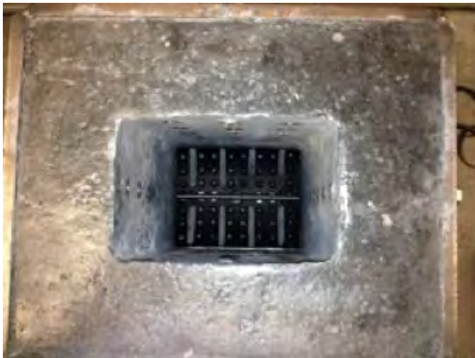
Figure 16. Inside of gasifier shell with refractory.
