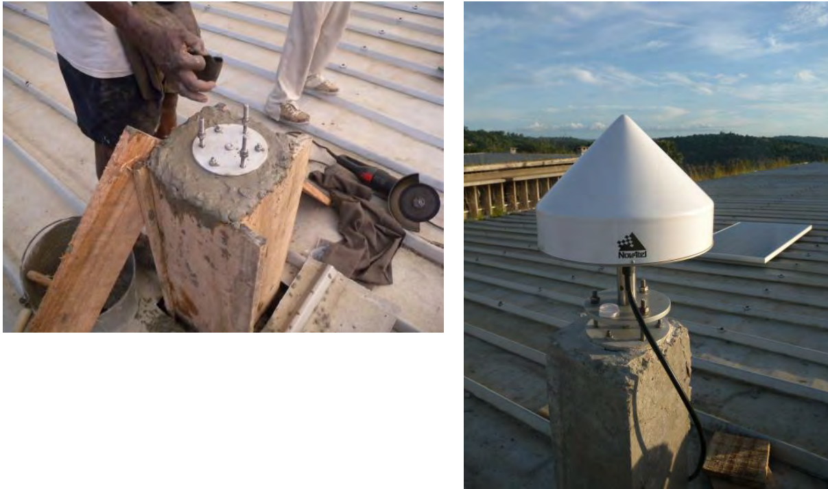
Figure 5 – Site FKIS (Kinshasa). Details of the antenna monument and ancillary equipment.
