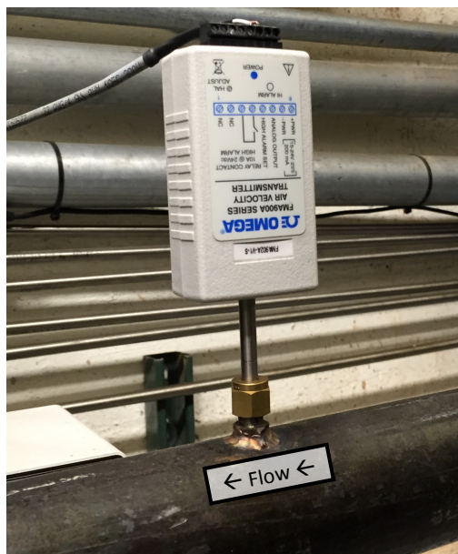
Figure 3.13. The intake pipe hot wire for intake mass flow measurements.
