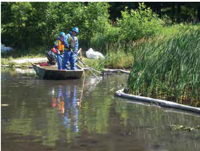
Crews use "stingers" to pump water into the sediment and flush oil to the surface. Photo courtesy of the EPA.
