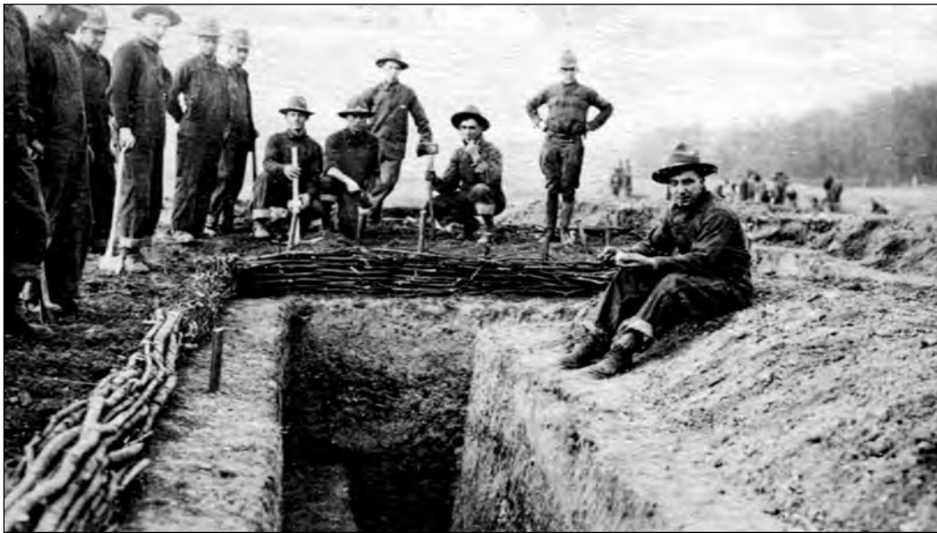
Figure 31. Completed trench at the Maneuver Grounds, circa 1918, post card by the Corte-Scope Co, Cleveland, Ohio (Beightler Armory, Columbus, Ohio).
