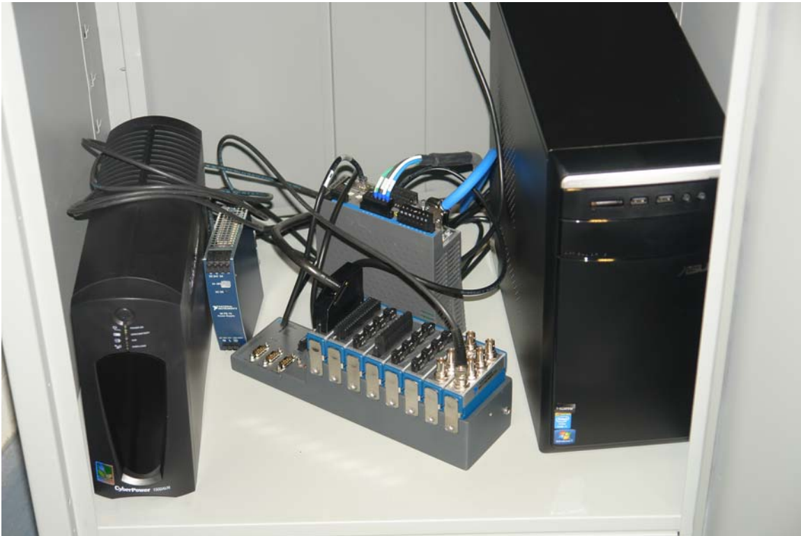
Figure 6. Shielded Faraday's cage for control electronics. From left to right: UPS power supply; 24-V power supply; NI cRIO 9068 real-time control module; Kollmorgen DDR servomotor interface; main control computer.
