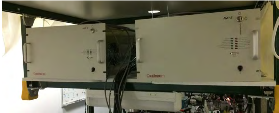
Figure 3: Two of the power supplies for the 19 mm diameter amplifiers
