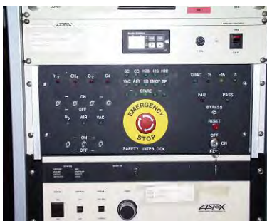
Figure A.34. Safety Interlock System
