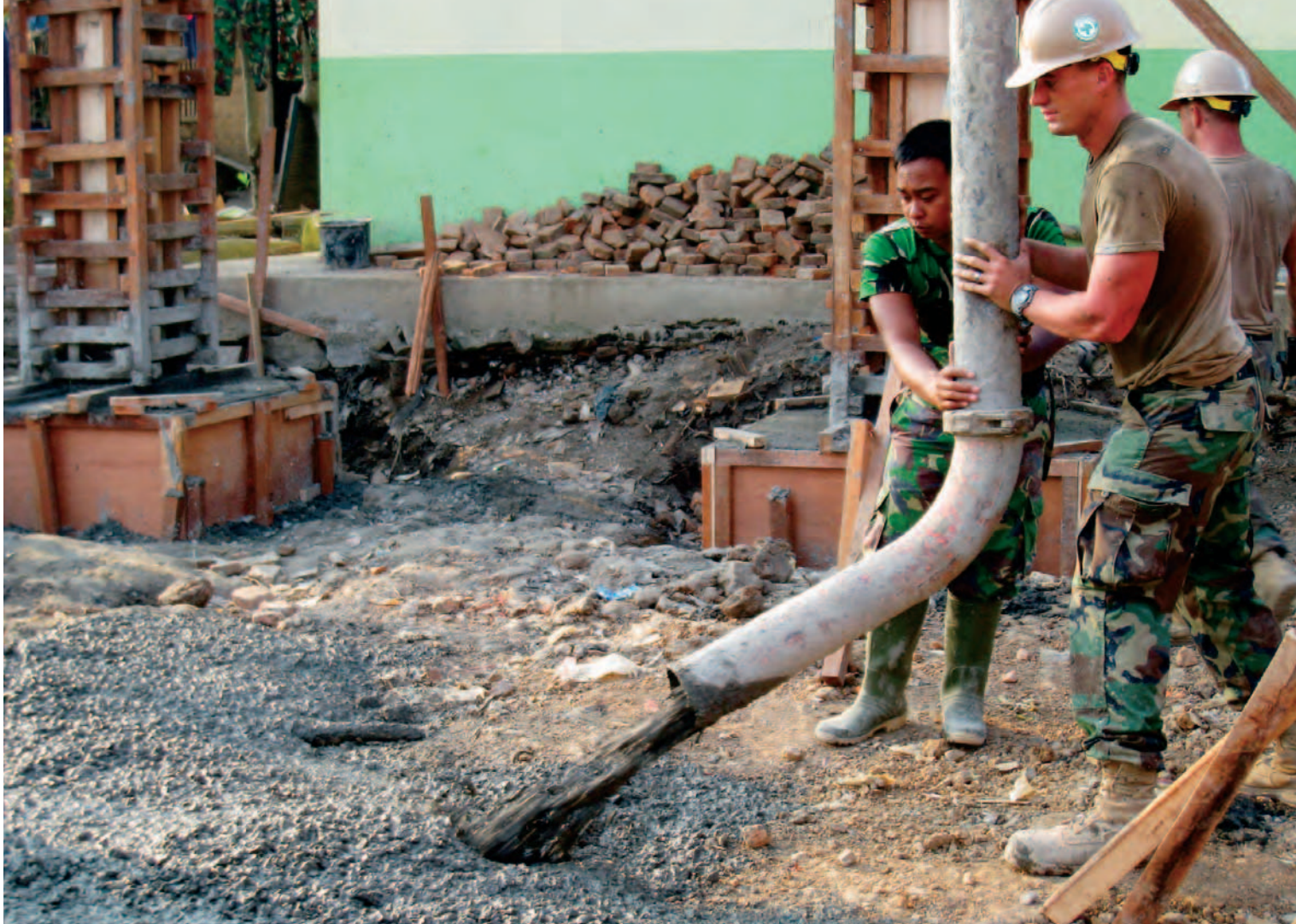
An Indonesian navy engineer and a U.S. Navy Seabee from Naval Mobile Construction Battalion 40 pour concrete for an engineering civic action program during the first phase of Cooperation Afloat Readiness and Training Indonesia 2009. Warfighters get the construction materials, fuel and other sustainment supplies they need during regular and humanitarian operations from the Defense Logistics Agency-Pacific Region team.
