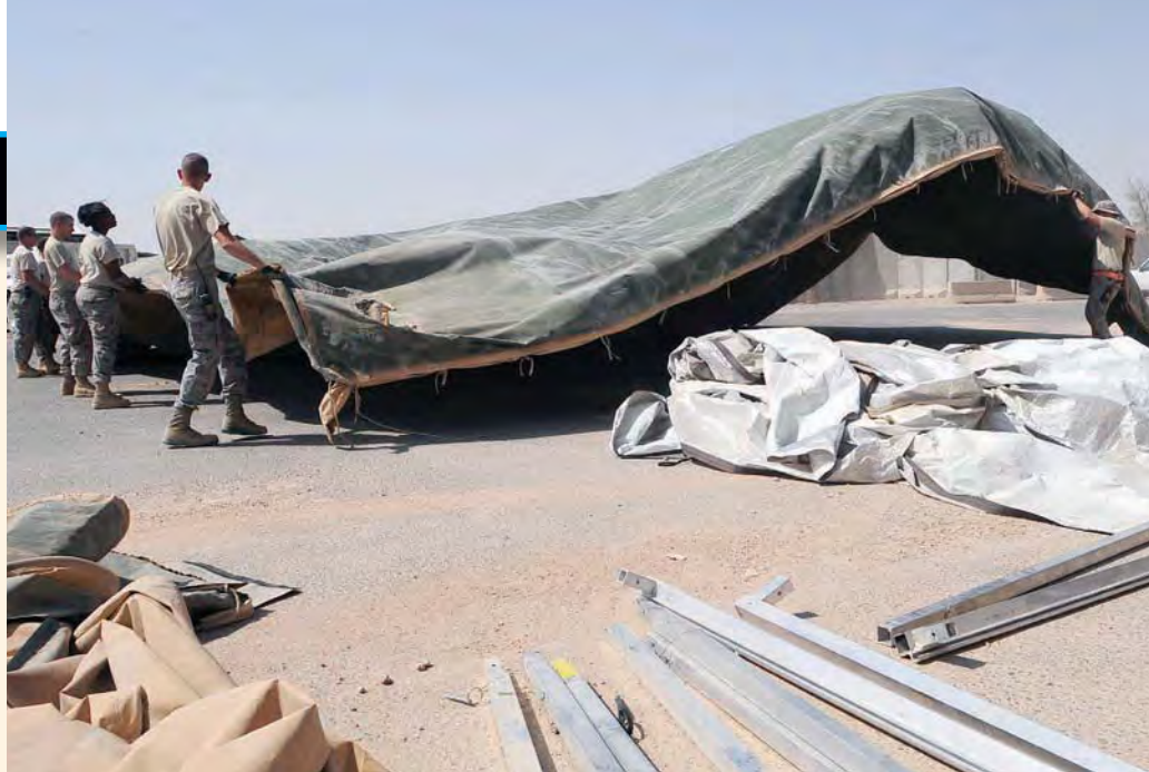
Air Force members of 407th Expeditionary Civil Engineer Squadron take down a tent structure. The squadron has been downsizing, which calls for consolidating material and equipment to send to U.S. warfighters in Afghanistan. A big piece of the Defense Logistics Agency’s mission involves the drawdown in Iraq and the reset of forces and supplies in Afghanistan.
