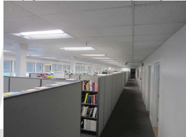
2'x4' lay-in LED luminaires
