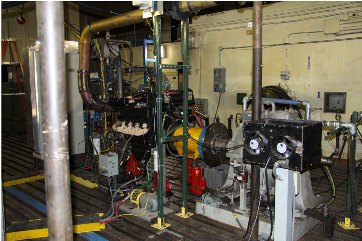
Figure 1: Cummins VTA903-T600, Bldg. 212, Cell 5
