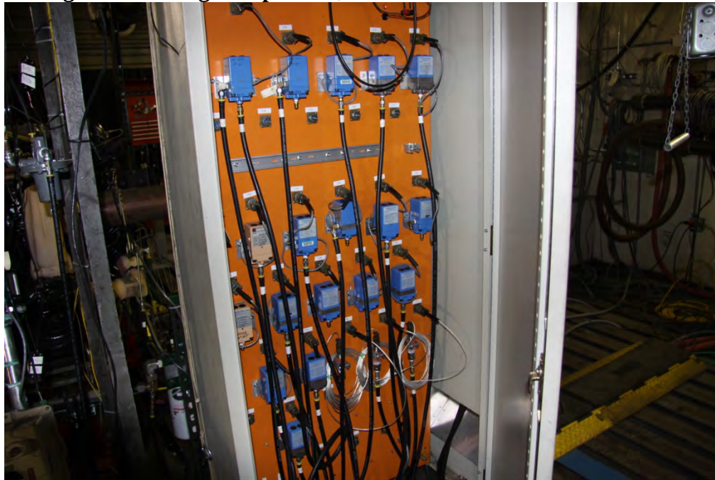
Figure 8: Testing Components, Pressure Transducer Cabinet
