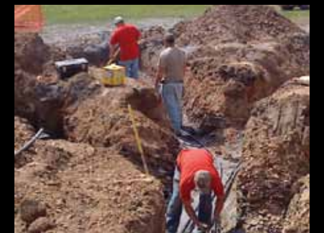
The NDCEE geothermal technology demonstration at Fort Indiantown Gap will help PANG achieve energy-independent facilities, one of its five strategic objectives for facility sustainability. This photo shows workers installing horizontal and vertical pipes for the heat pump system.
