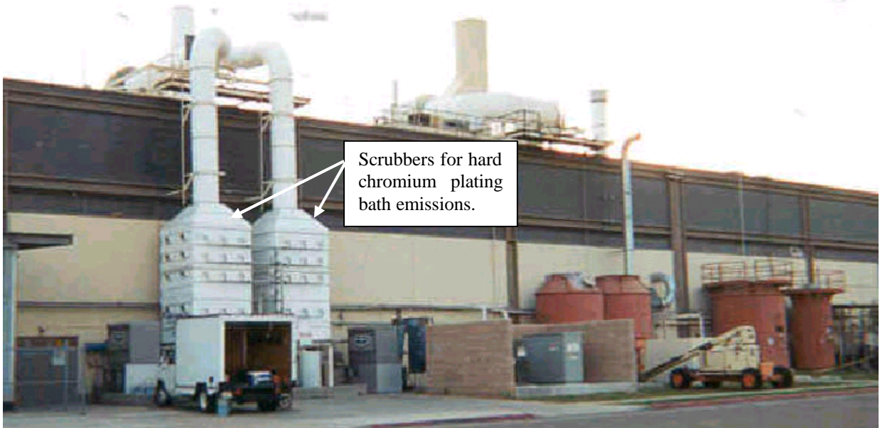
Figure 9 – NORTH ISLAND FUME SCRUBBERS
