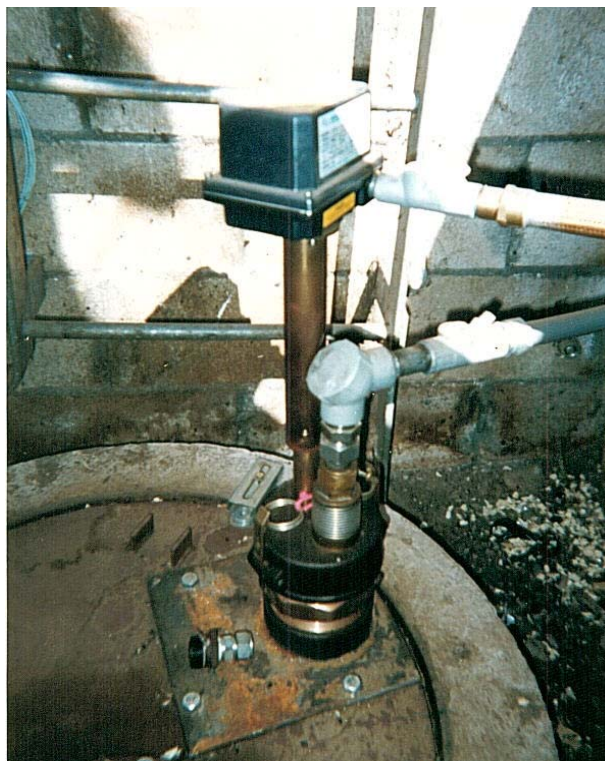
Figure 9. Mounting system for a permanently installed LRDP in a bulk UST.
