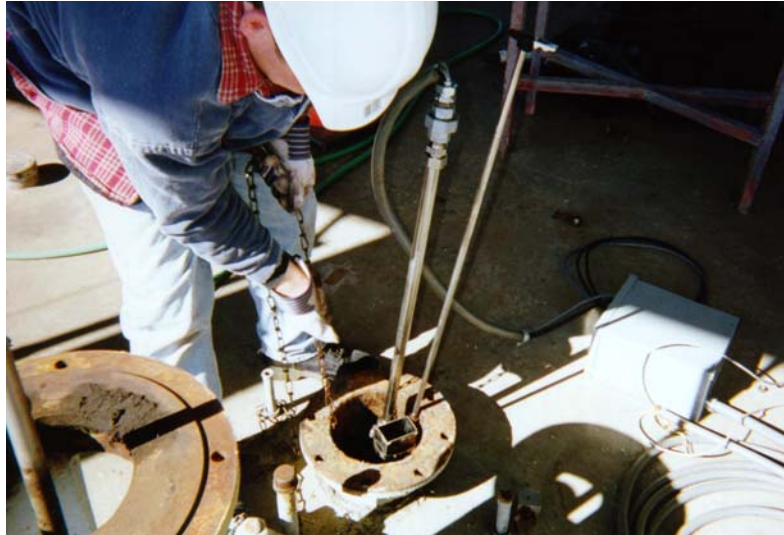
Figure 18. Top of the being installed in an 8-in. opening in a 50,000-gal UST.
