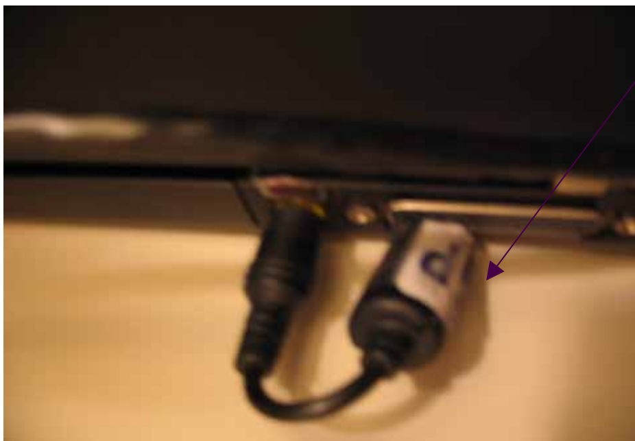
Server Power Cable from Server to Outlet
