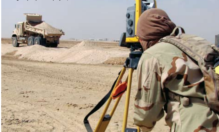
Navy engineer surveys elevation of dirt added to landing strip expansion project, Helmand Province
