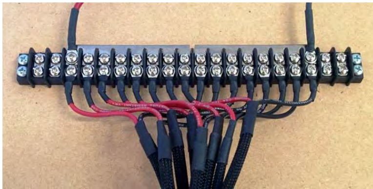
Figure 16. Power distribution terminal block
