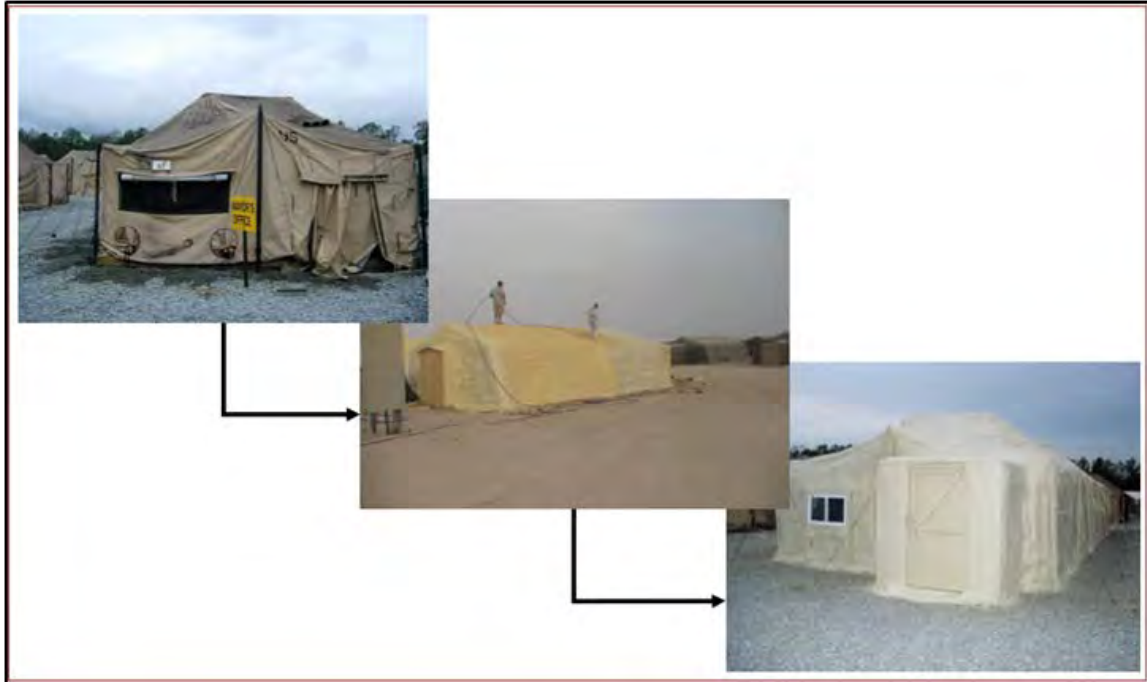
Figure 2. General-purpose-medium (GP-M) tent before, during, and after closed-cell foam insulation application (from Foulkner & Wilke, 2010).
