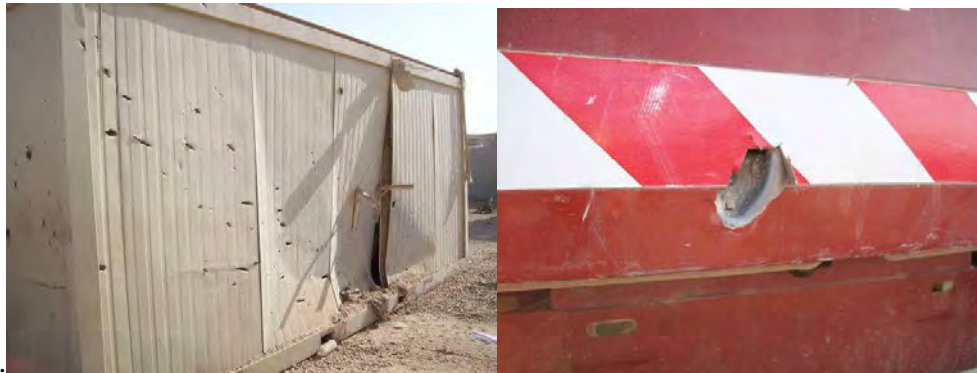
Figure 5. Damage to a metal building and the tailgate of a pick-up truck approximately 50 yards from the impact site of the 107mm rocket (from Mason Knowles Consulting LLC, 2015).
