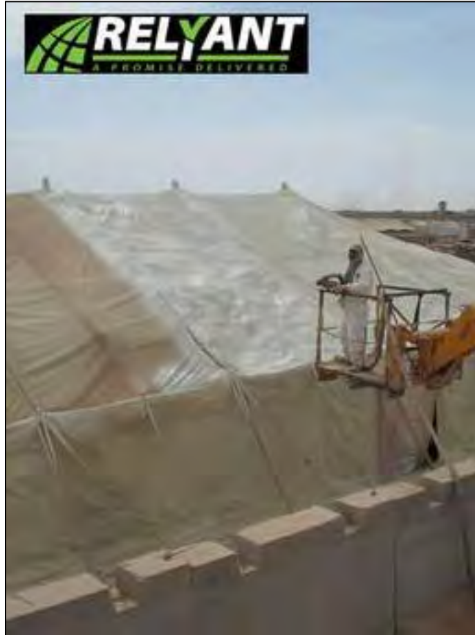
Figure 14. Relyant, LLC employee applies spray foam insulation to a tent structure in Afghanistan (from Sprayfoam.com Inc., 2010).
