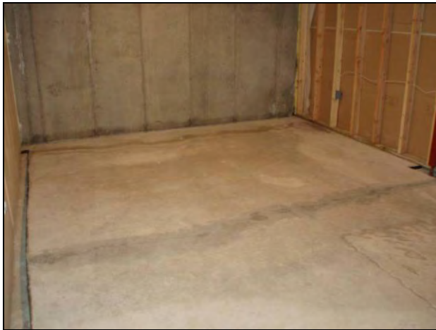
Figure 2-4. Foundational Issues at Minuteman Village Requiring Renovation/Demolition
