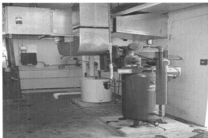
Mechanical Room Figure 1-3
