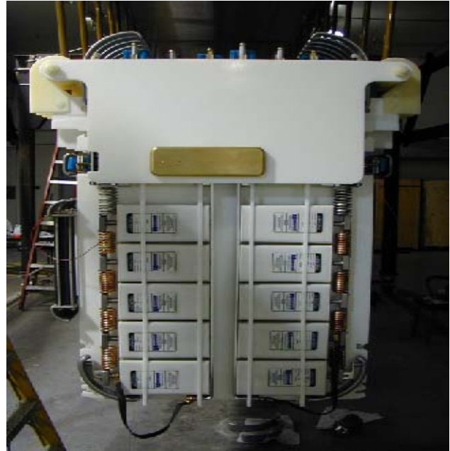
Figure 6. End view of Marx with second capacitors of Gibbs section missing.
