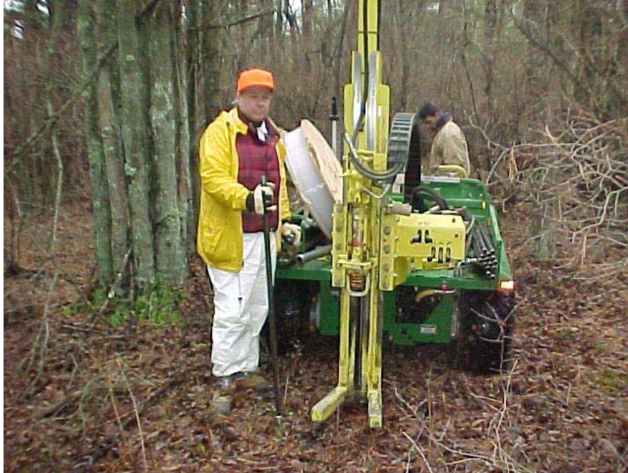
Figure 2.7. Direct push GeoProbe rig mounted onto a John Deere Gator. This drill rig was used at the Colliers Mills WMA wetland site at McGuire AFB, NJ to obtain sediment cores and install drive-point piezometers.
