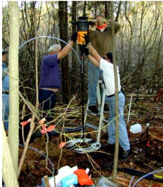
Figure 4.12. Installation of narrow diameter drive-point piezometer using percussion hammer. Note the Teflon tubing inner sleeve extruding out of the hammer adapter. The Teflon tubing is connected by tubing barb to a stainless-steel drive-point tip with screens for ground-water inflow (Solinst Canada Ltd.).
