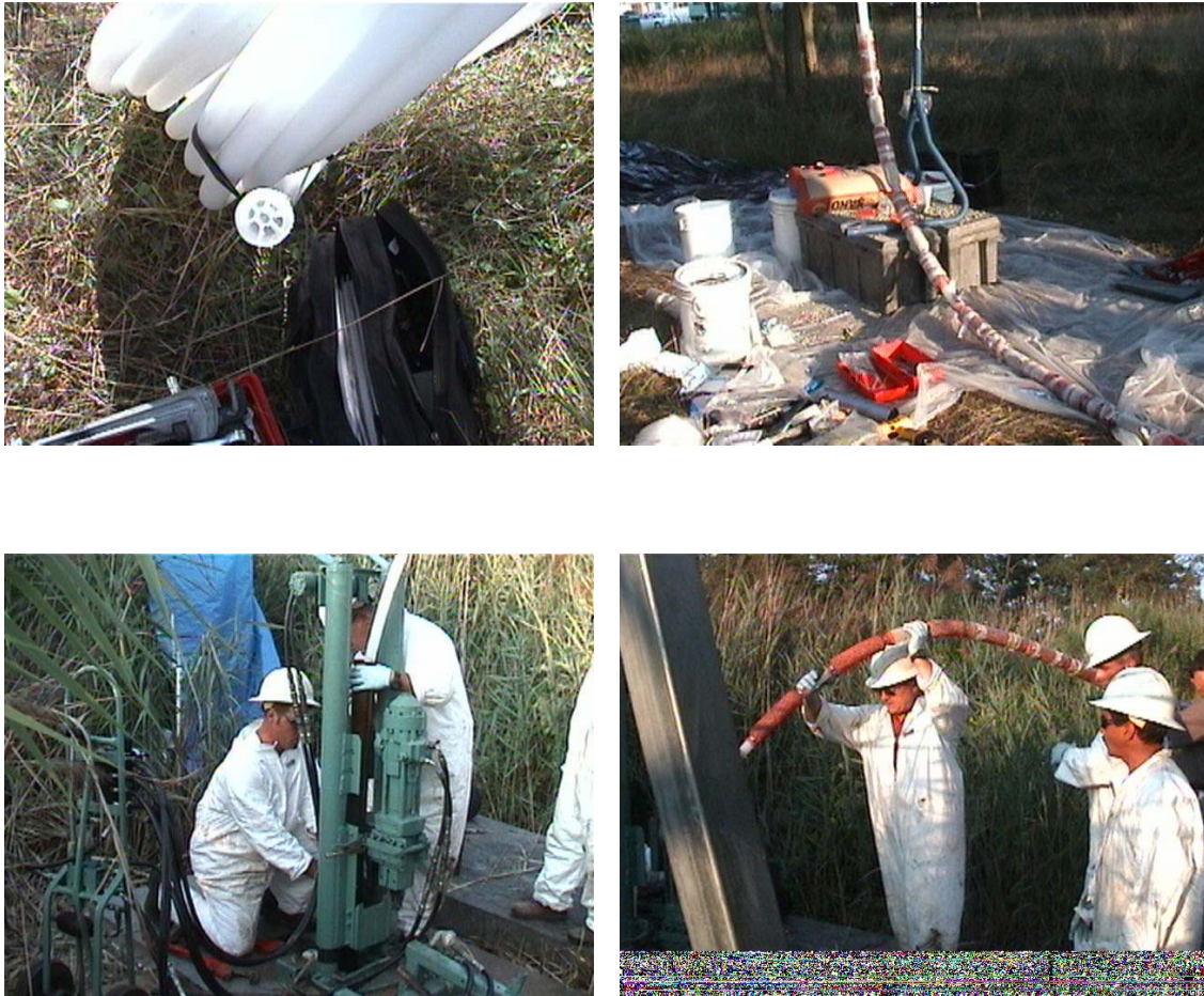
Figure 4.20. Preparation and installation of Multi-Level Monitoring System (MLMS; Precision Sampling, Inc.) at wetland study site: (A) coiled 7-chamber polyethylene tubing, (B) preparation of MLMS with sand packers and bentonite packers, (C) drilling of borehole with vibratory rig; and (D) insertion of MLMS down borehole casing. The borehole casing is immediately removed upon insertion of MLMS.
