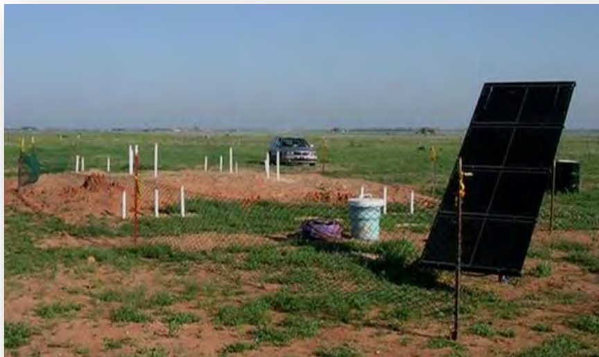
Solar-powered in situ bioreactor, Altus AFB, OK
