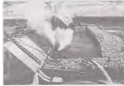
Completed cofferdam at Dam No. 14 with two of the concrete monoliths in place. When the steam pump removes water from inside the cofferdam, building the remaining monoliths will begin.
