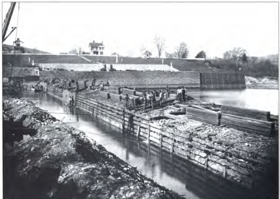
Timbercrib dams were constructed by framing pens resembling log cabins, setting them side by side across the river, then filling them with stone and planking the top.
