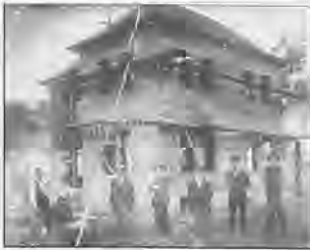
Lock house under construction for the resident lock keeper (lockmaster) and his family.
