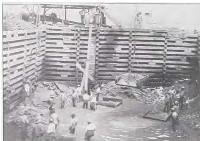
Men shovel muck inside a cofferdam into skips for hoisting and removal while a steam pump in the background removes the water.
