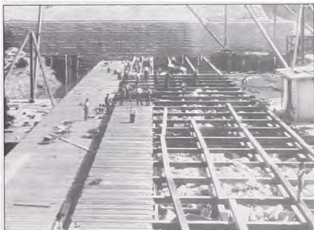
Building the timbercrib dam at No. 7, showing the stone-filled cribs before they were planked over.
