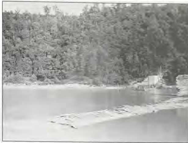
View of Dam No. 5 showing the breach in the dam.
