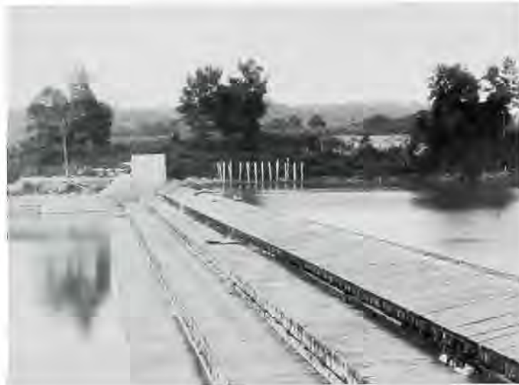
The finished timbercrib dams were planked over and stepped down like a staircase.
