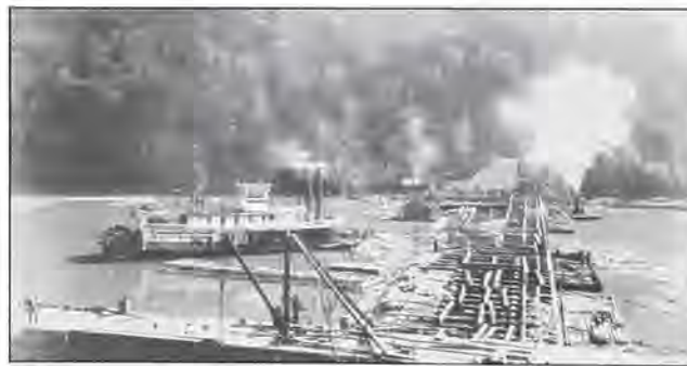
The steamboat Grace Morris assists with the construction of a timbercrib dam.
