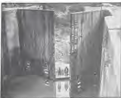
Lock No. 5's deteriorated lockgates in 1885.
