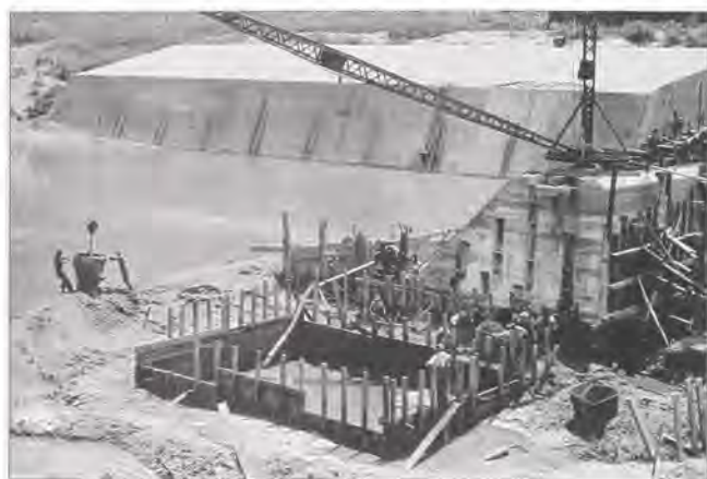
Building forms for a concrete monolith at Dam No. 13 in Aug. 1914. The derrick and bucket is placing earth to raise the temporary cofferdam.
