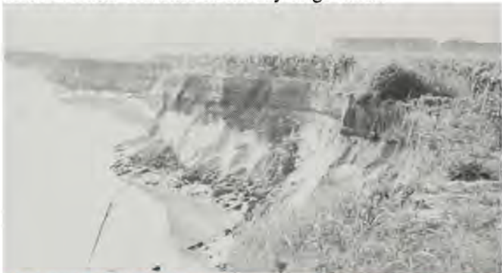
ILLUSTRATION 30. Eroded Arkansas River bank at Pine Bluff.
