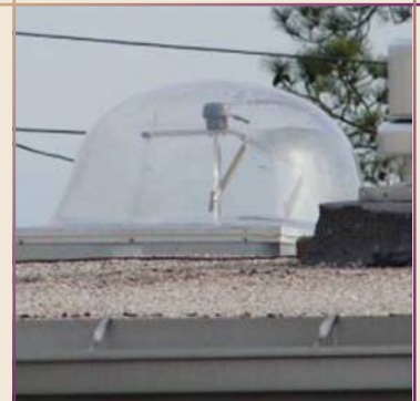
The dome, mirror, and tracking mechanism of a daylighting system is mounted on the roof of a building at Fort Bragg, NC. A solar cell powers the tracking mechanism that controls the mirrors to optimize the sunlight transmitted to the lobby below.
