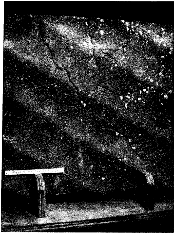
Figure 1. Typical "cracked" concrete slab.
