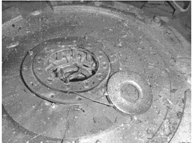
Figure 4. Typical damage to load region.
