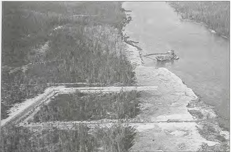
Dredge excavates on the east bank of the Atchafalaya River (1965). The ring levee in the center of the photograph protects a cemetery.
