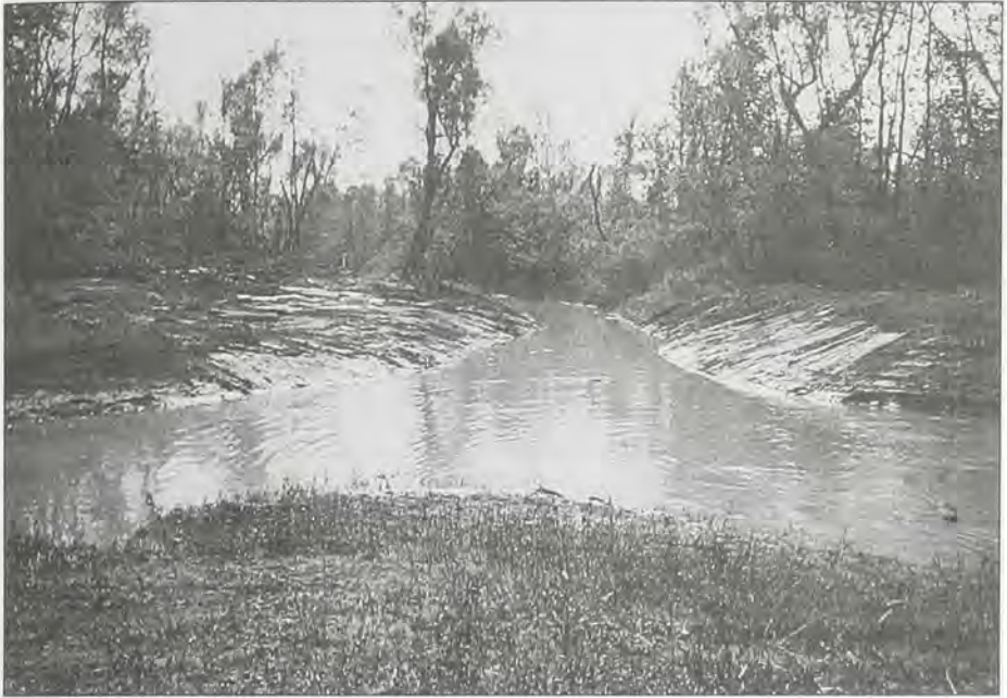
Demonstration project in Buffalo Cove management unit. V-cut construction with snagging and clearing at Bayou Eugene, November 1994.
