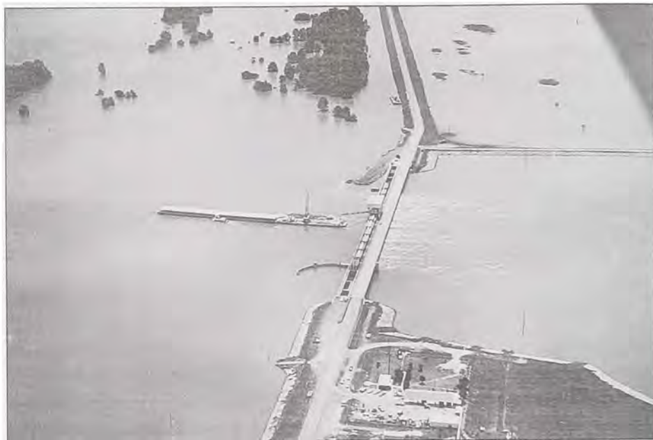
The low sill structure during the 1973 flood and after the collapse of one wingwall on the inflow side (just above the center of the photograph).
