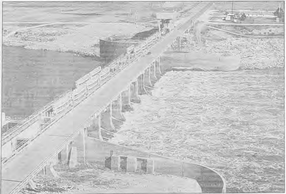
Low sill structure before the wingwall failure.
