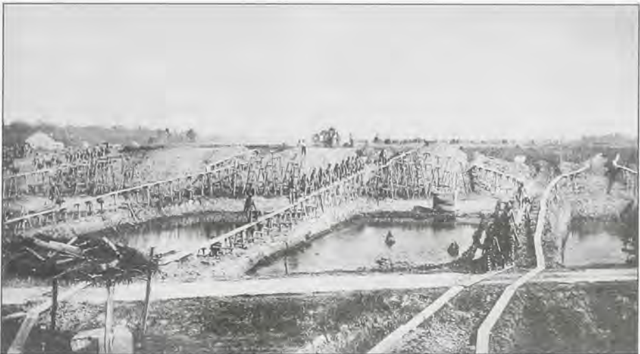
Prisoners use wheelbarrows to construct a levee in 1890 to close the Morganza Crevasse about 25 miles below Old River.
