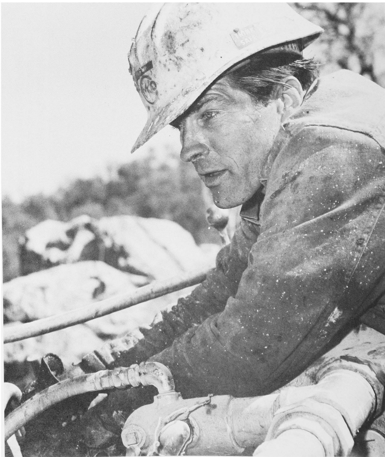
A POWDER MONKEY TAKES A BREATHER DURING A HARD DAY'S WORK AT THE NEW MELONES DAMSITE.
