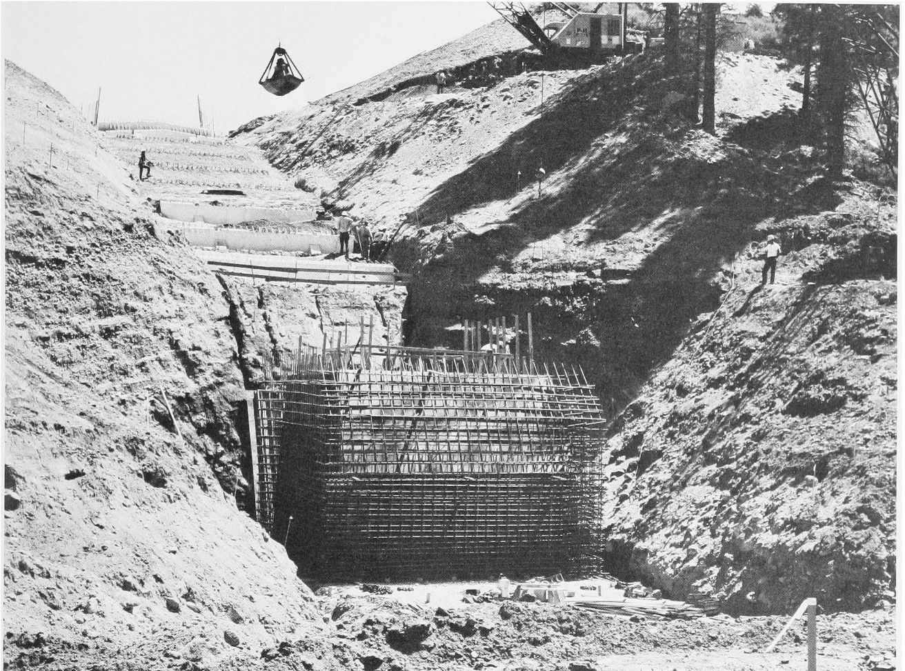
THE SPILLWAY OF THE MARTIS CREEK DAM, UNDER CONSTRUCTION BY THE PERINI CORPORATION FOR THE SACRAMENTO DISTRICT, CORPS OF ENGINEERS. PHOTO TAKE 26 AUGUST 1970.
