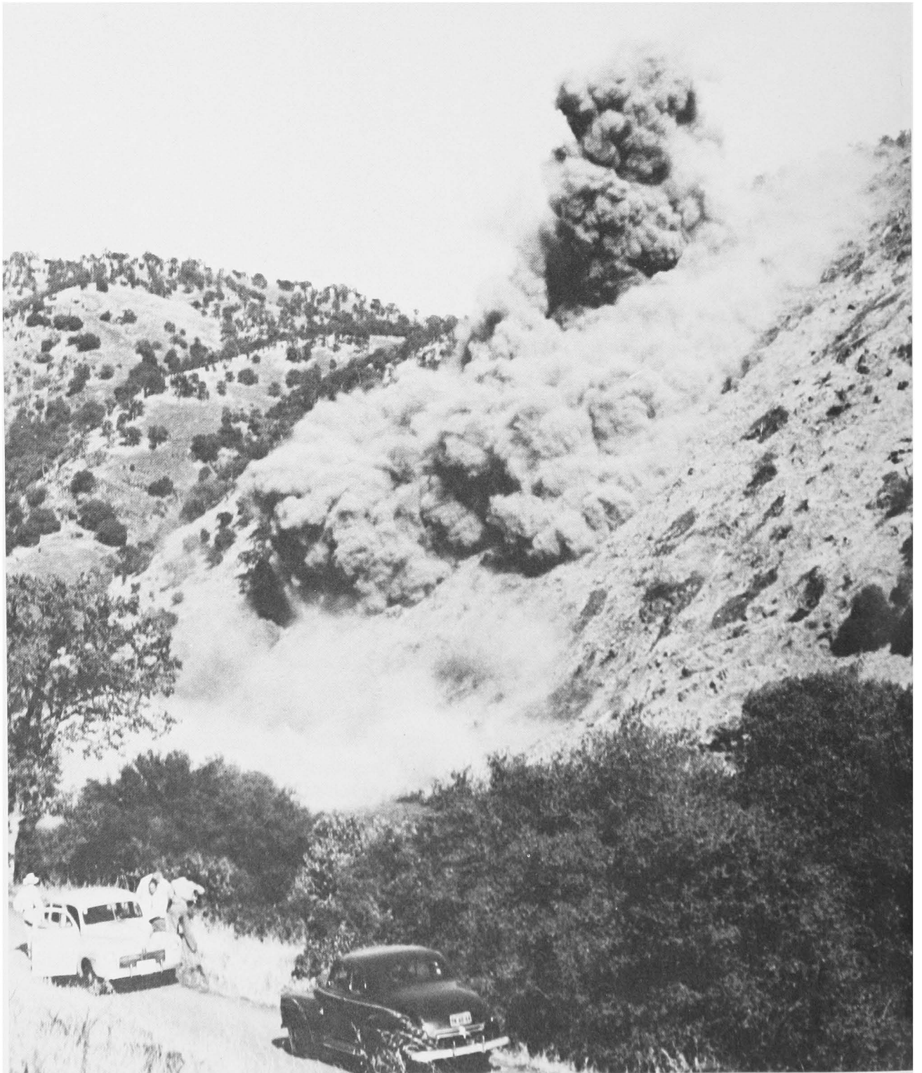
GOVERNOR WARREN SET OFF THE FIRST BLAST TO MARK THE BEGINNING OF CONSTRUCTION OF PINE FLAT DAM — MAY 27, 1947
