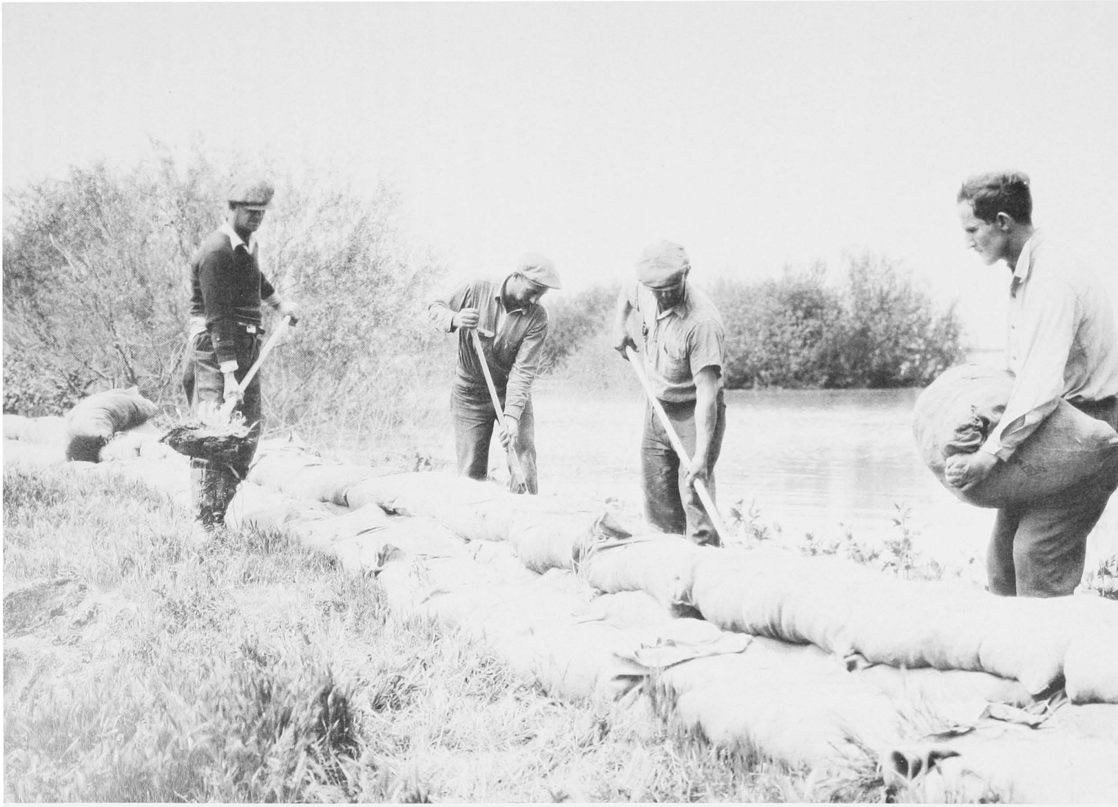
MEN WORKED HARD AND LONG DURING THE THIRTIES TO REINFORCE LEVEES ALONG THE SACRAMENTO AND SAN JOAQUIN RIVERS.
