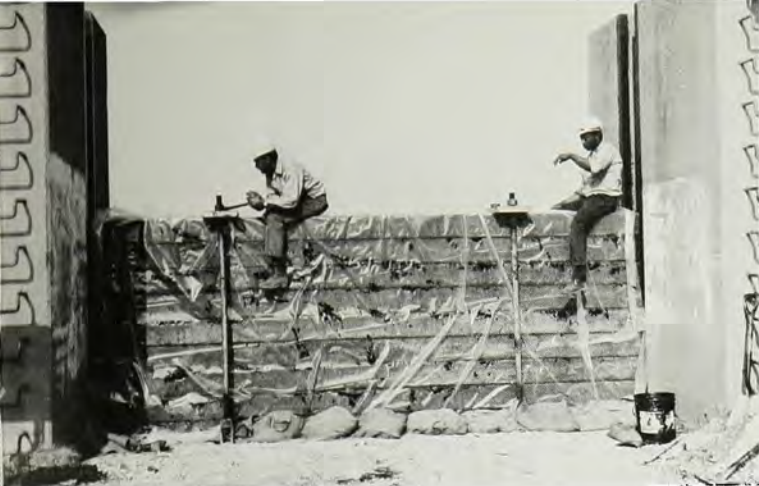
Highwater 1975 - Fourth Street Gate Closure, Cairo, Illinois.
